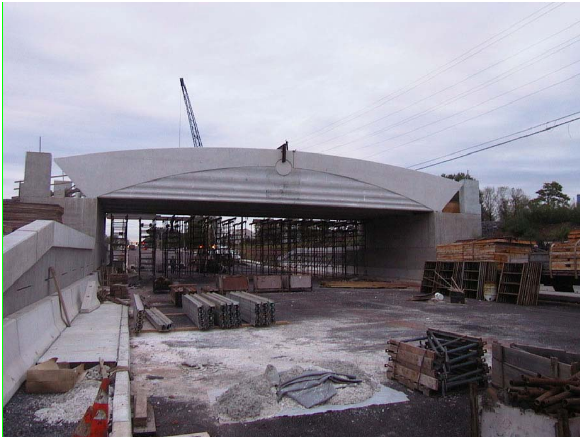
Figure 6 – Forty Foot Road was excavated and utilities relocated. The contractor elected to build the roadway base course and erect scaffolding to support structural formwork for the fascia beams. The fascia beams were designed with haunches to bear the outer edges of the deck. Three interior stringer beams support a traditional structural concrete deck. Computer-cut foam art forms were used inside the structural forms to create the fascia art motif. Structural pylons were clad with formed concrete art panels.
