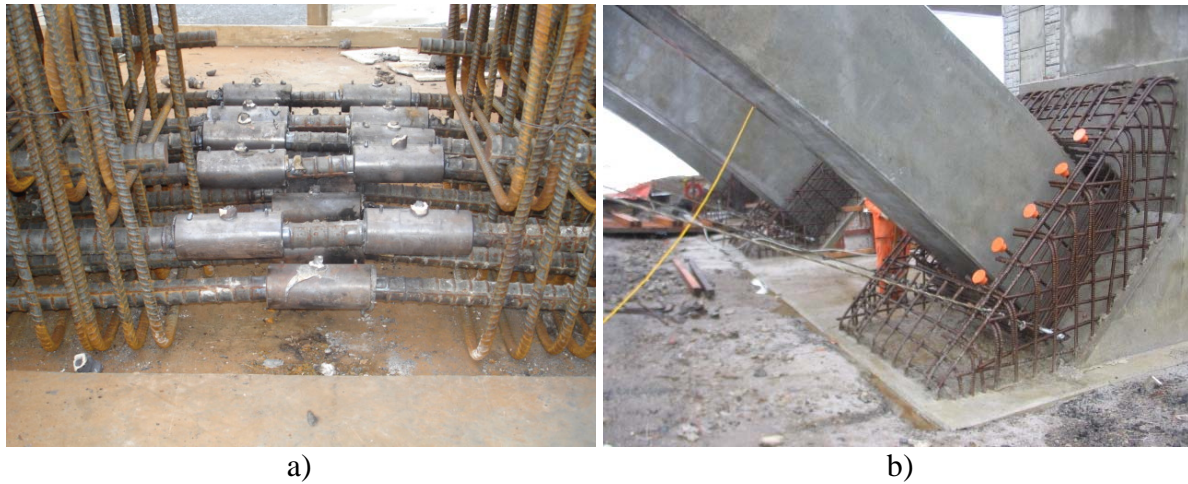
Fig. 6 – a) Mechanical Splices for Arch Reinforcing Steel; b) Arch Socket Reinforcing Cage
