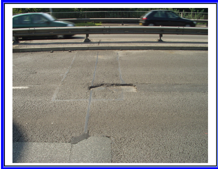
Failure of surfacing at joint in bridge
