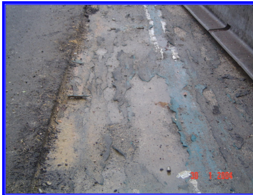
Unbonded membrane easily removed
