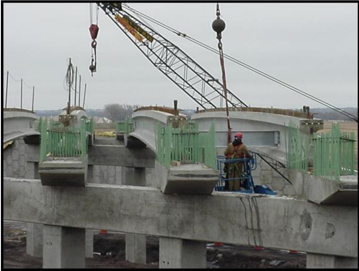
Fig. 6 Visible camber in Clarks Bridge, Clarks, NE, due to extended time between prestress release and erection
