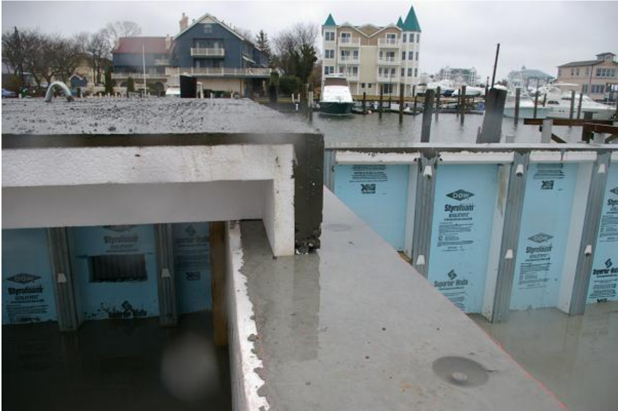
Fig. 3 One side of the floor panel mounted on top of bearing wall.
