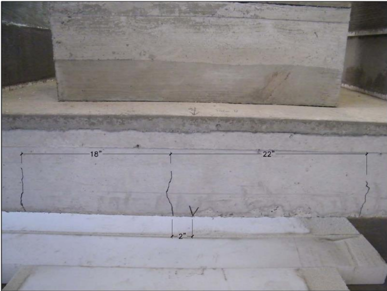
Fig. 13 Cracking at mid-span after step 6
