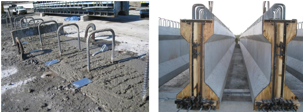
Figure 1 - Top Surface of Girder after Finishing and Girders after Removal from Bed
