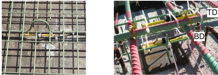
(a) PC/PS panels (b) CIP deck Fig. 4. VWSG installation details (panels and deck)
