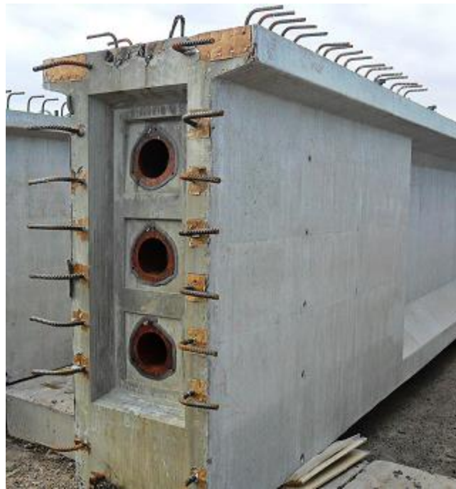
Figure 16 – PT Anchors at Precast Girder End Block (Photo by Jason Kuck, Tpac)
