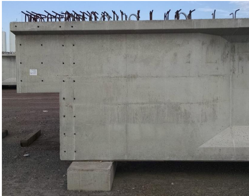
Figure 20 – Dapped End Detail at Span 3 Precast Girders (Photo by Jason Kuck, Tpac)
