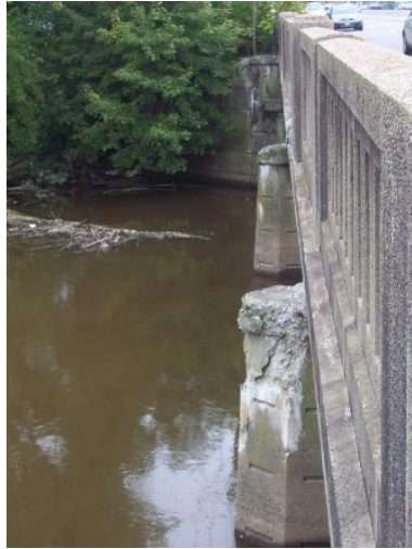
Photo 3 - Deteriorated bridge seats at abutments and piers.
