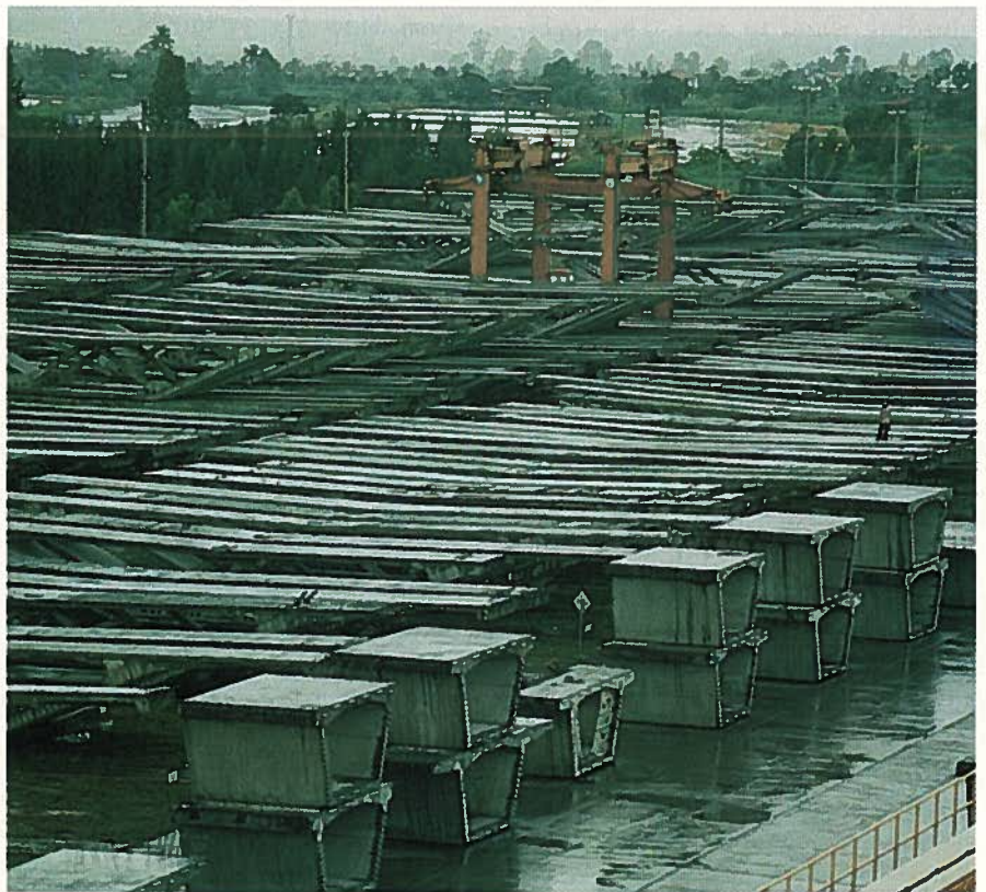
Fig. 14. Storage area for D6 and D2/D3 segments.
