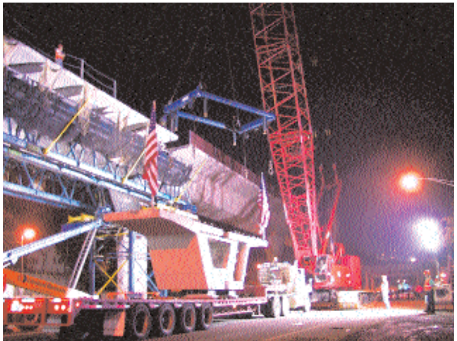
Fig. 1. This night-time photo shows erection of the last precast concrete segment – three months ahead of schedule. Photo courtesy: Figg Engineering Group.
