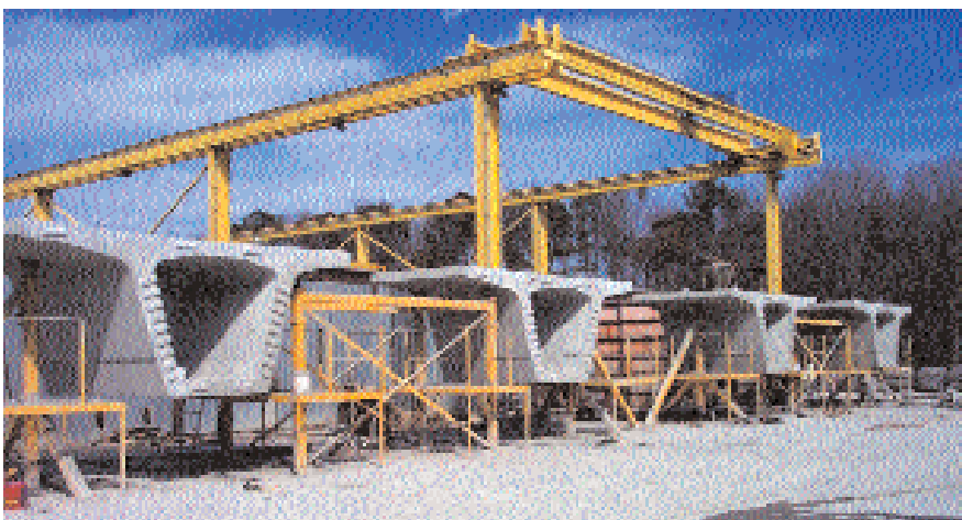
Fig. 10. Bayshore's casting cells (single-track segments shown) were set up with waiting positions in which segments were prepared for storage after being removed from the match-cast position. Photo courtesy: Bayshore Concrete Products.
