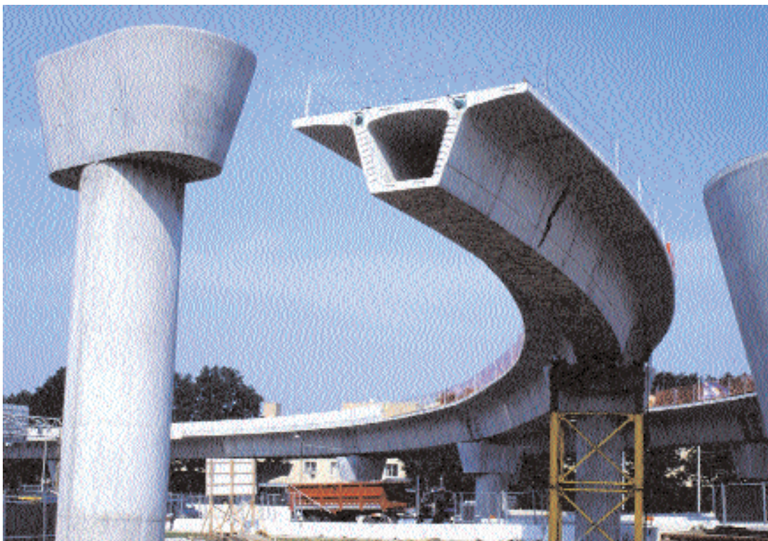
Fig. 7. In areas with tight curvatures, spans were constructed in a balanced cantilever method. Balanced cantilever construction was used on about 50 of the 474 spans of the AirTrain project. Photo courtesy: Figg Engineering Group.
