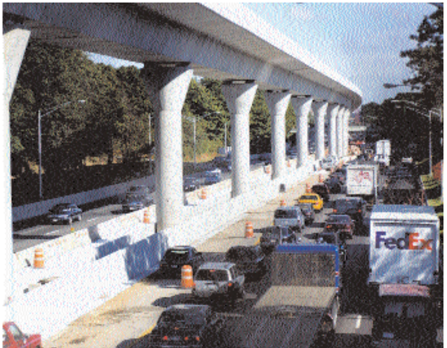
Fig. 2. The Van Wyck Expressway offered very limited space in which to construct a light rail system. Beyond the challenge of erecting the superstructure in a very restricted space, three lanes of traffic on either side of the rail line had to be maintained during the course of the project. Photo courtesy: Figg Engineering Group.
