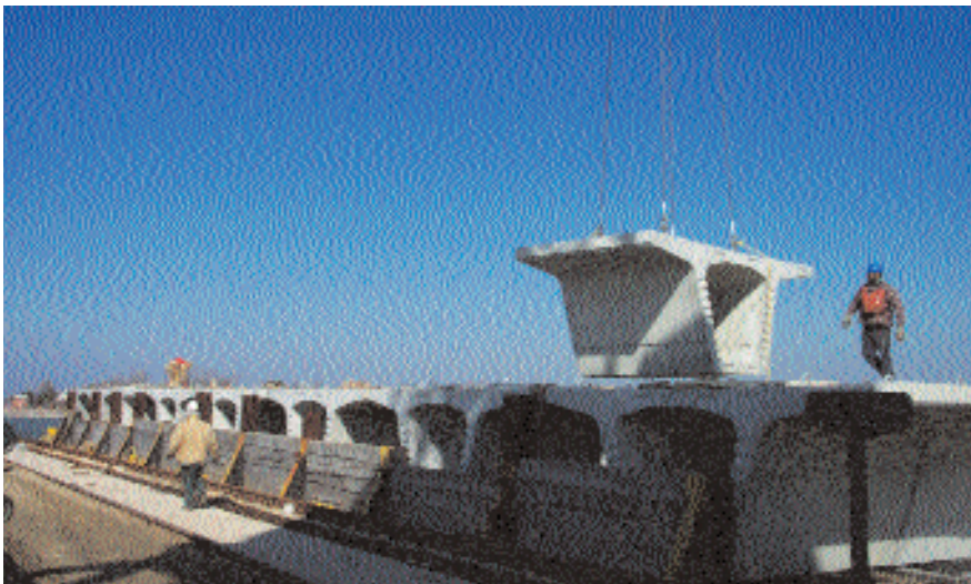
Fig. 13. After casting, the segments were barged 250 miles (402 km) before being transferred to a low-boy tractor-trailer for the 100 mile (161 km) trip to the site. Photo courtesy: Bayshore Concrete Products.
