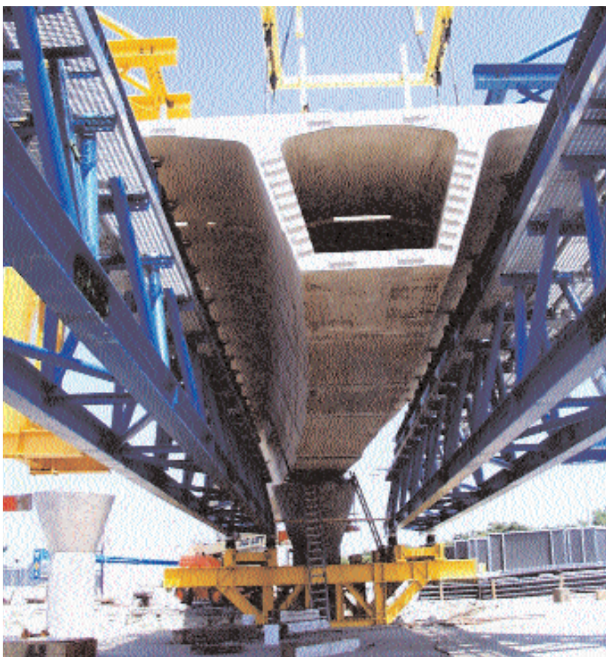
Fig. 17. The truss design consisted of two different types of trusses, one for Type 1 precast segments, and the other to accommodate the loading requirements of both Type 1 and Type 2 segments. Photo courtesy: Figg Engineering Group.
