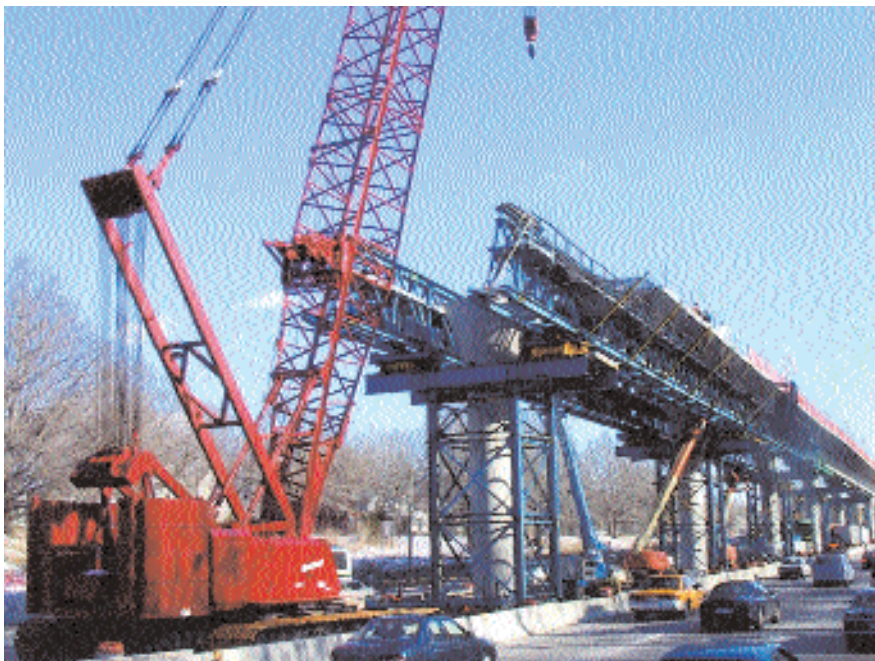
Fig. 16. The guideway management team was faced with developing an erection system that would accommodate the different span configurations, be able to negotiate problematic radii on curves, and function in an extremely restricted area. Photo courtesy: Figg Engineering Group.
