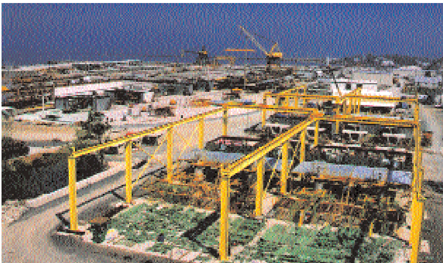
Fig. 9. Bayshore added $7 million in casting facilities to produce the different precast products required for the AirTrain System. The casting facilities encompassed a large portion of the 85 acre (34 ha) Virginia facility. Photo courtesy: Bayshore Concrete Products.
