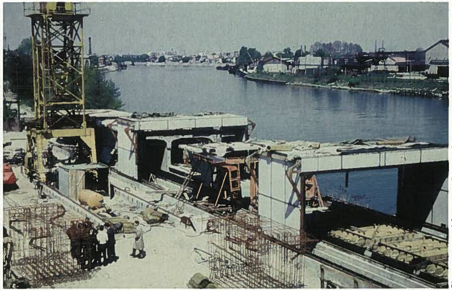
Fig. 7. Shown is the long-bed precasting at the Choisy-le-Roi site in Paris, France.
