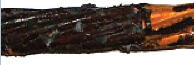
Figure 18. This strand from the macrocell corrosion test series was removed from the beam in Fig. 3, which experienced longitudinal cracking thereby facilitating severe corrosion of the strand.
