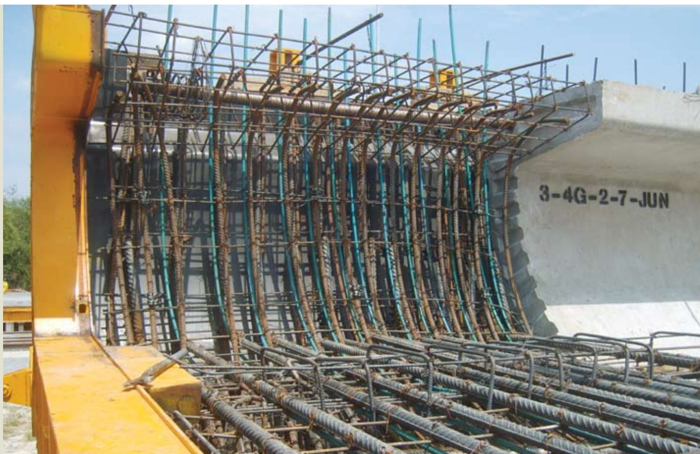
Figure 13. The pier segments were cast against their associated typical segment in a short bed.
