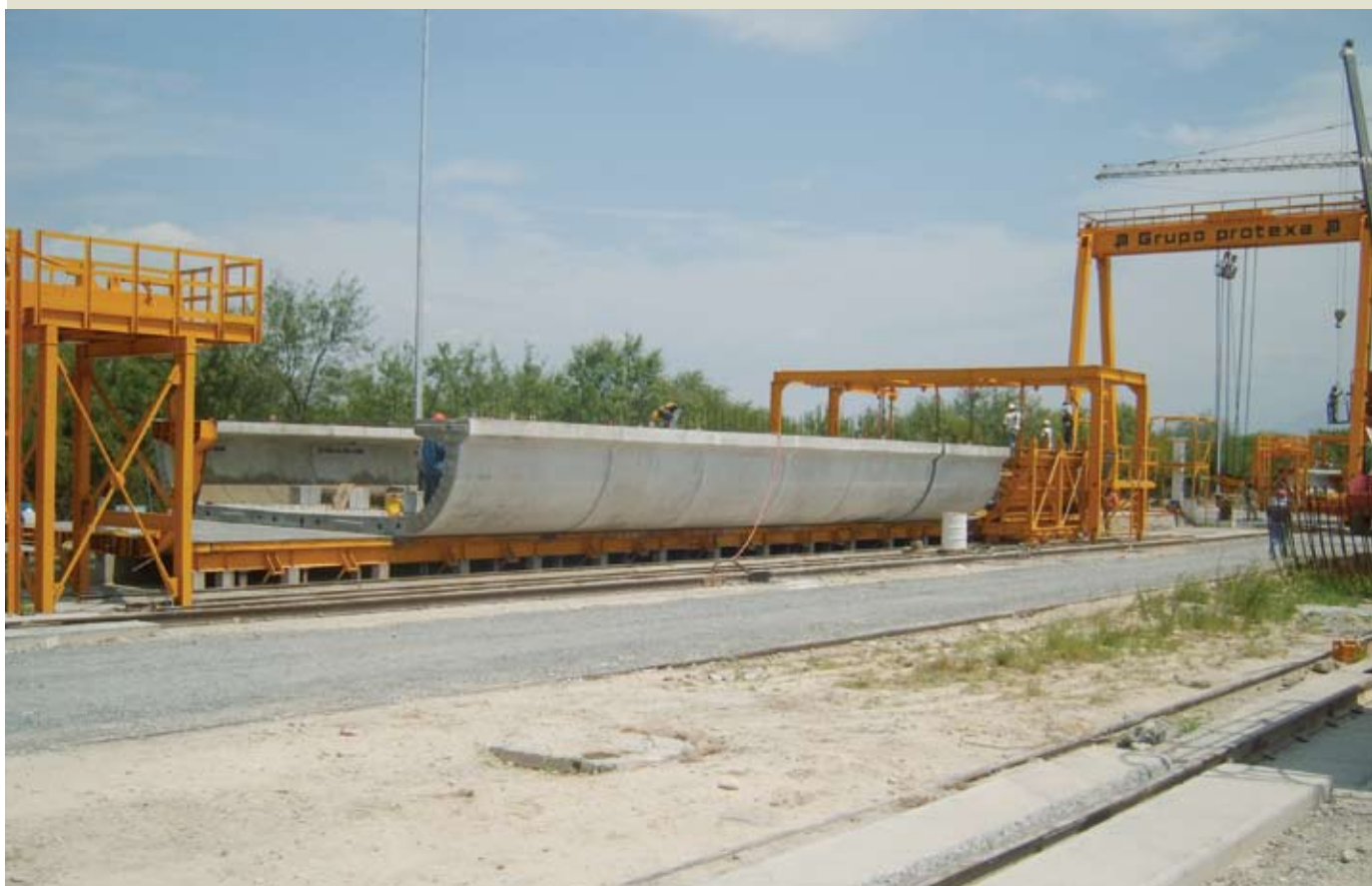
Figure 12. The shape of the cross section and the use of greased and sheathed strands simplified both the casting forms and the labor needed to cast and stress the tendons.
