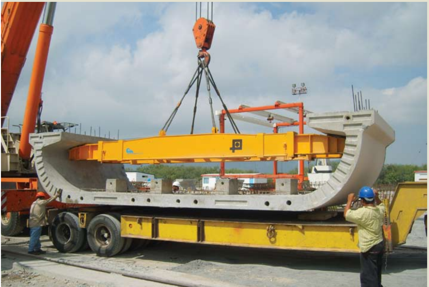
Figure 6. This photo shows a typical segment with a clear view of the cross section.
