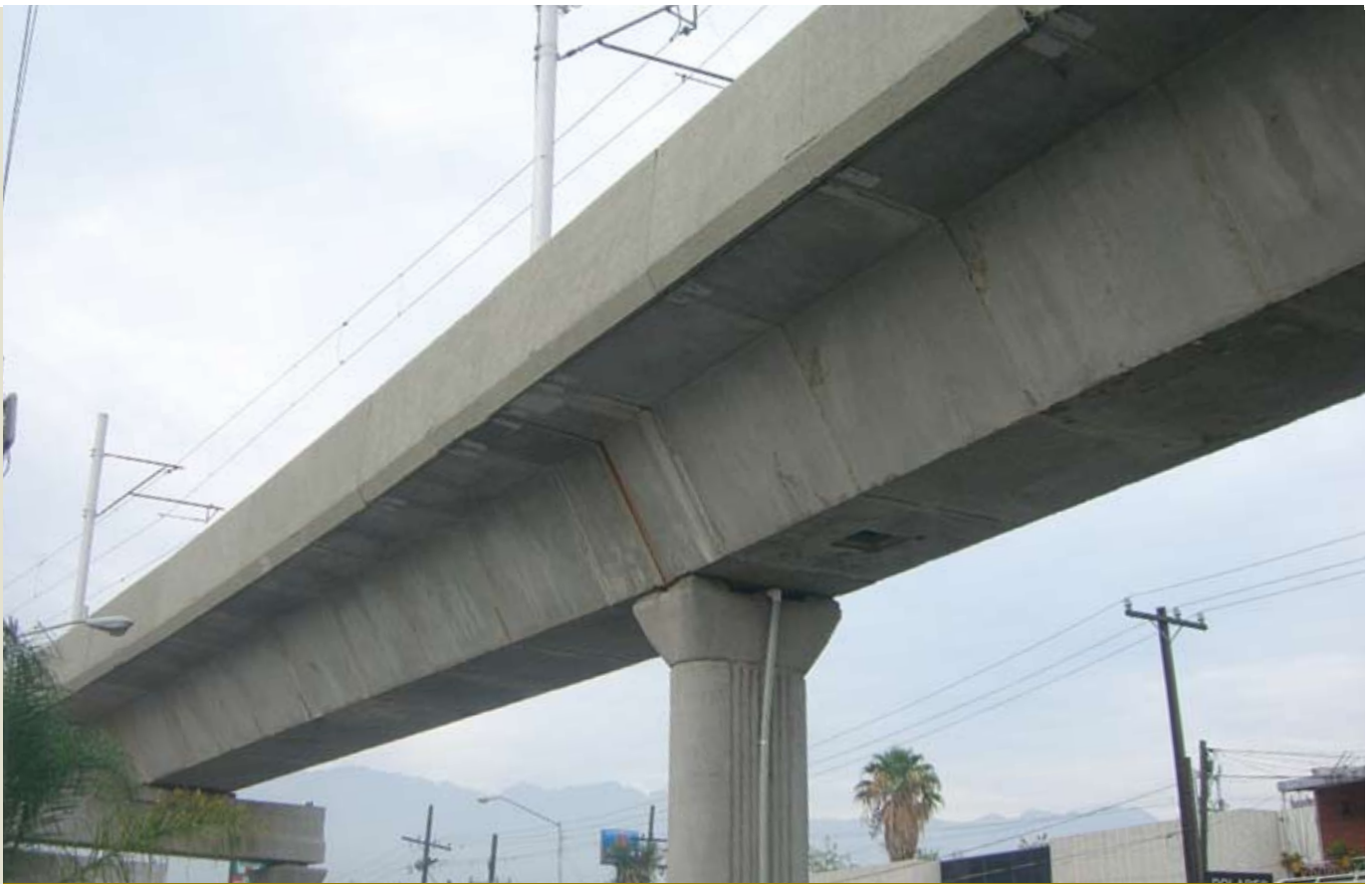
Figure 1. The precast concrete segmental structure used for the Metrorrey linea 1 concrete segmental viaduct was designed by the late Jean Muller.
