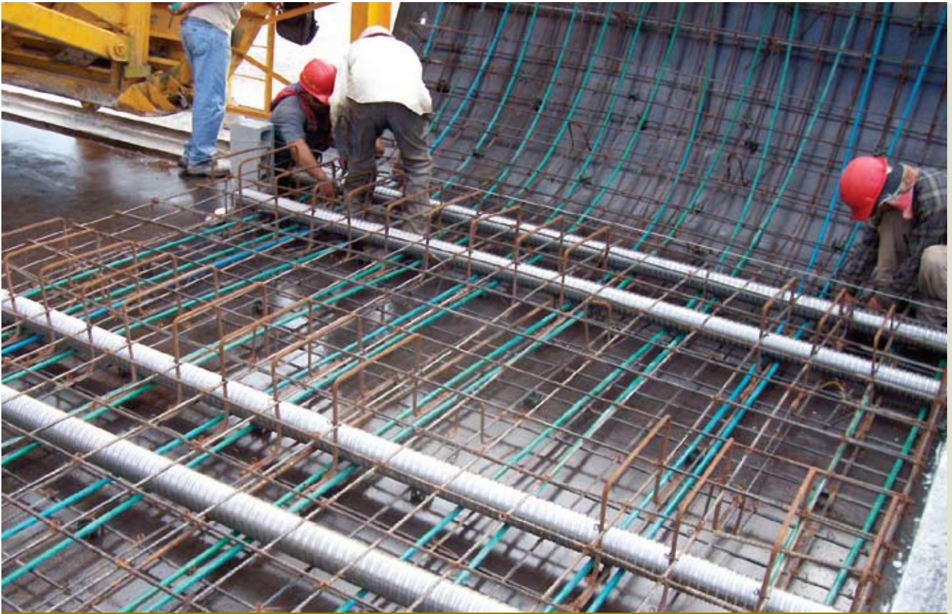
Figure 8. A typical segment of the Metrorrey linea 2 contains 10M (no. 3) reinforcing bars at a spacing of about 220 mm (8.7 in.) across the entire surface of the cross section.
