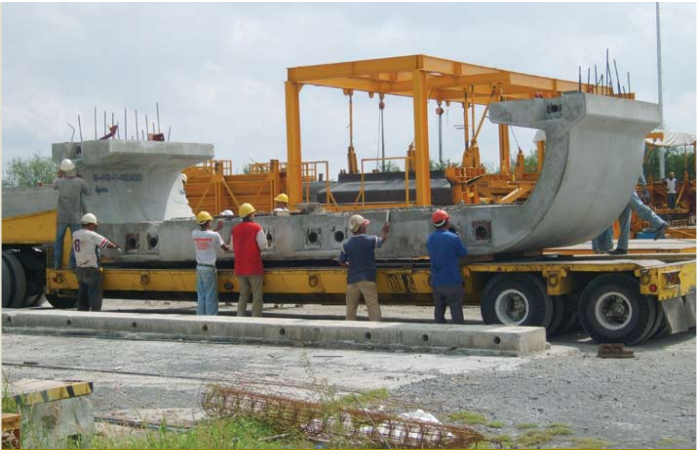
Figure 7. This photo shows the typical pier segment and highlights some of the anchoring.
