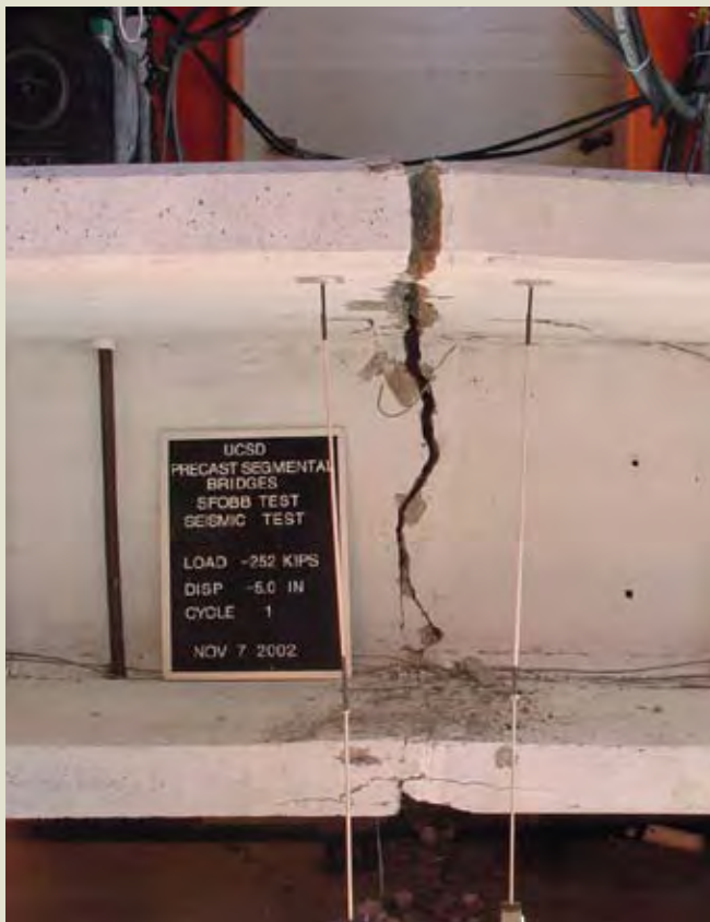
Test unit 100INT-AUXT rupture of deck auxiliary tendons
