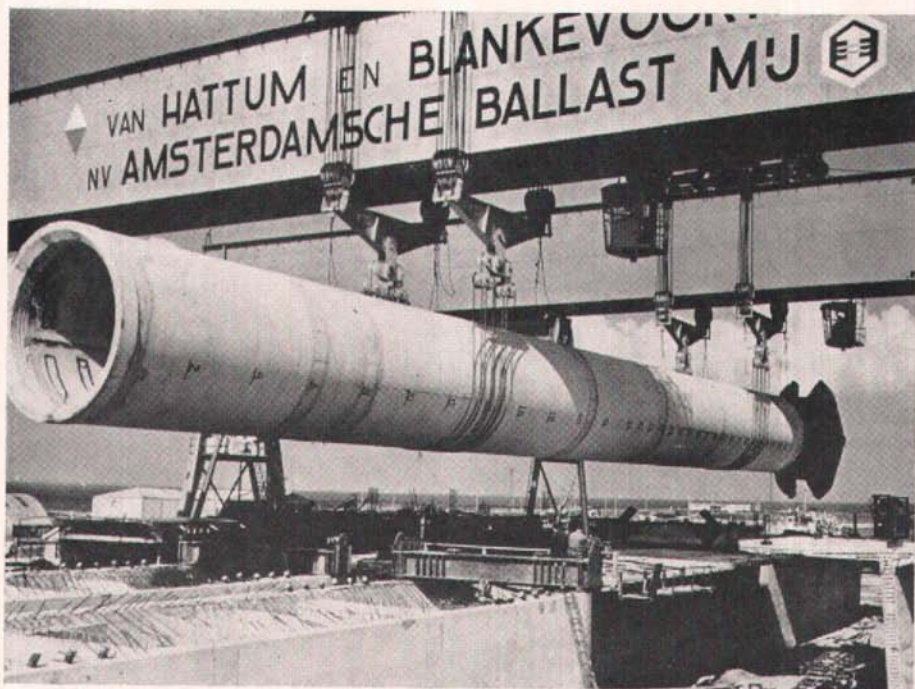
Fig. 3—A prestressed cylinder pile, 14 ft. in diameter and 120 ft. in length, being loaded out from casting yard
