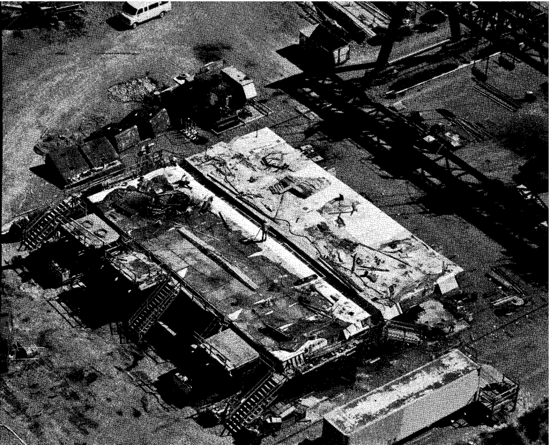
Fig. 8. Girder element match-casting site. The 80-ft (24 m) element on the left is in a stationary steel form.
