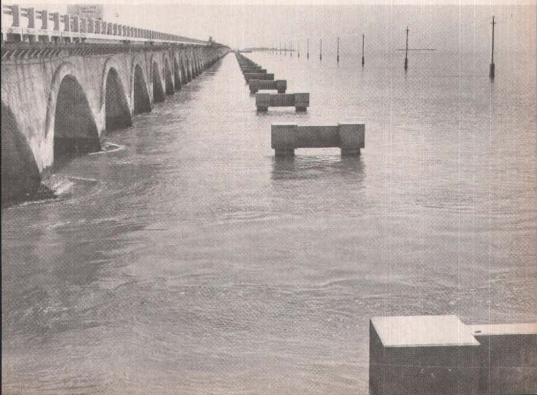
Fig. 12. Precast struts join the tops of two piles by being cast integrally with a cast-in-place cap. V-piers bear on top of caps.
