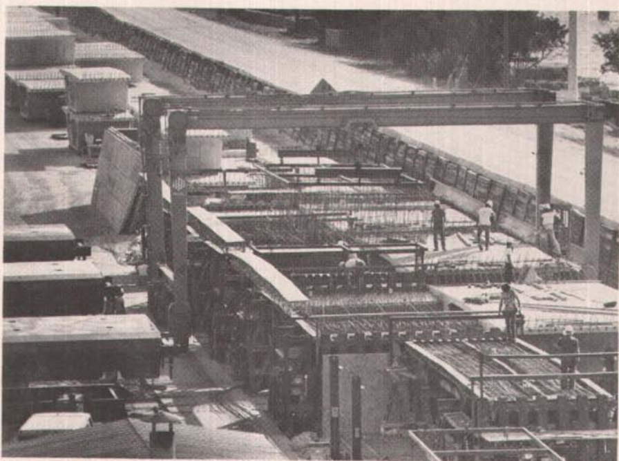
Fig. 7. Casting yard. Typical scene every morning when reinforcing steel is being placed in the new box girder segments. The precast elements were produced by the short line method in four casting machines.
