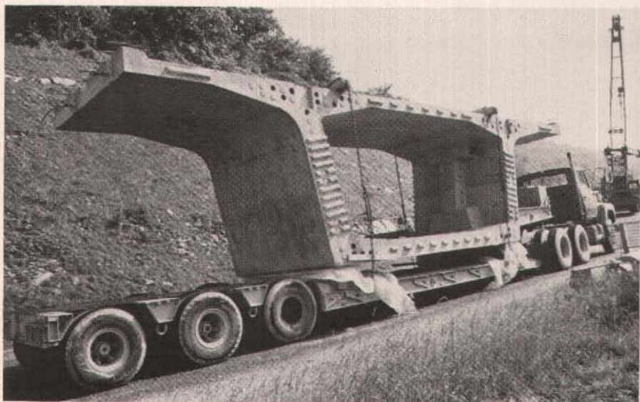
One of the 9 ft (2.75 m) deep precast segments for Linn Cove Viaduct being trucked to construction site. The segments were cast inside a building about a mile (1.6 km) from bridge. Indoor casting was necessary due to severe weather of the Blue Ridge Mountain region of North Carolina.
