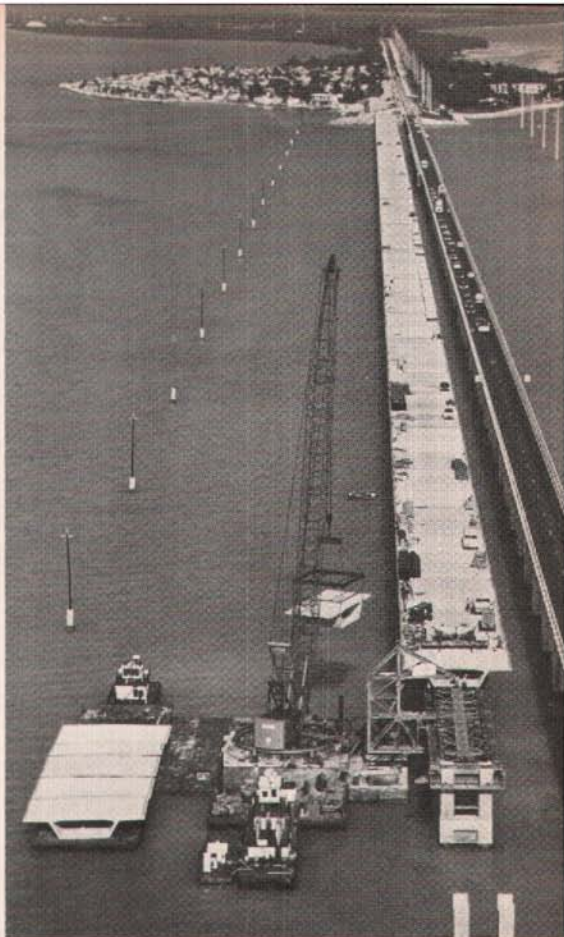
Aerial view of completed portion of 12,144 ft (3704 m) Long Key Bridge. Contractor has been able to place five spans in one week—590 ft (180 m) of completed bridge deck.
