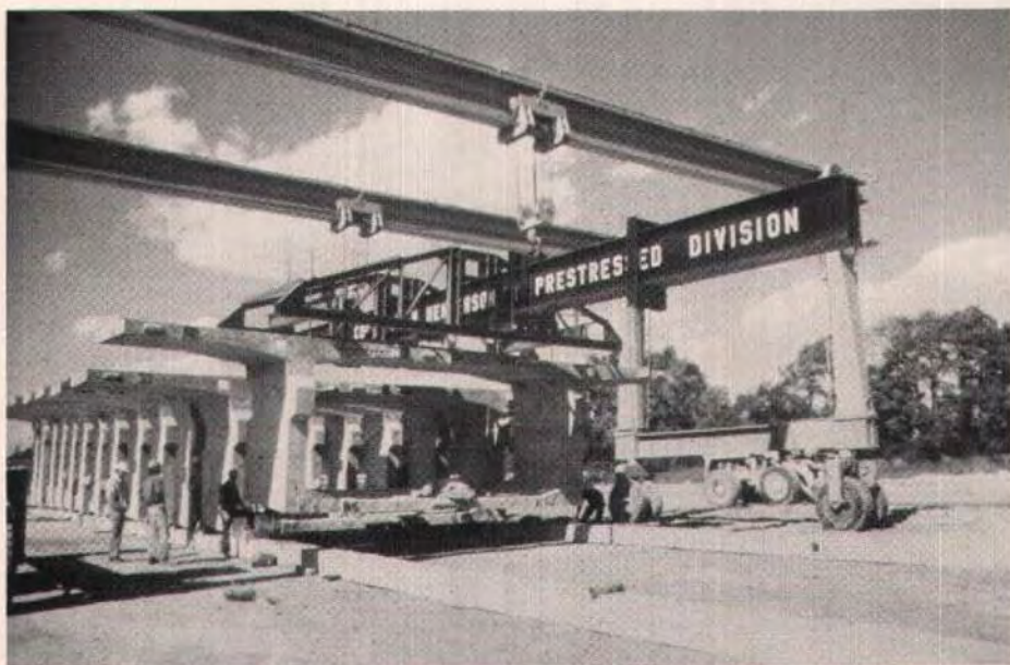
Fig. 15. Once the length of the bed was produced the segments were stored in the yard to await delivery.
