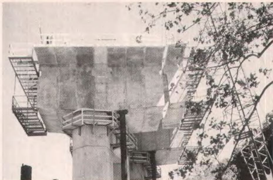
Fig. 20. Erection continued from the pier in each direction always keeping within one segment of balanced cantilevers.
