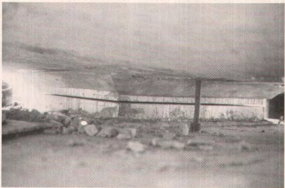
Fig. 24. The pot bearings were grouted in place after the balanced cantilevers were lined up.
