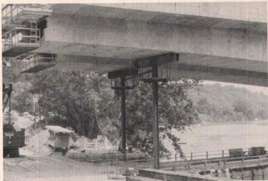
Fig. 25. An erection strut was placed in each end span to stabilize the cantilevers.
