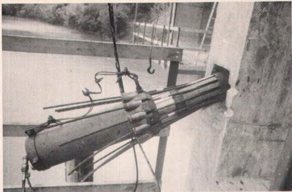
Fig. 21. The hydraulic jack, shown here pulling draped tendons in the web wall, tensioned twelve ½-in. (13 mm) diameter 270K strands and had a piston to seat the anchorage cone.
