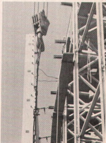
Fig. 4c. Precast panel being readied into position on tank wall. Note connecting dowels on side of panel.
