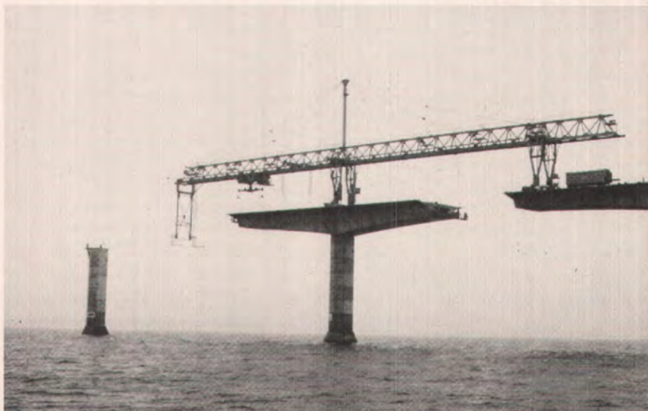
Fig. 14. Balanced cantilever construction employing a launching girder at the Sallingsund Bridge, Denmark.
