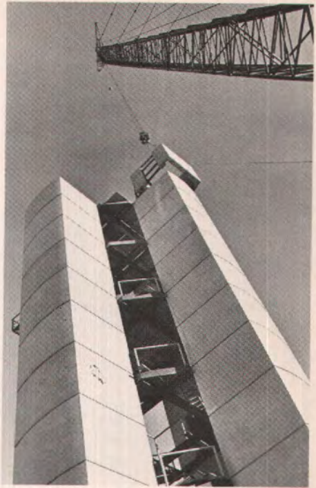
Fig. 1(b). Erection of precast box segments. Note that the modules were stacked to 180-ft (54.9 m) height.
