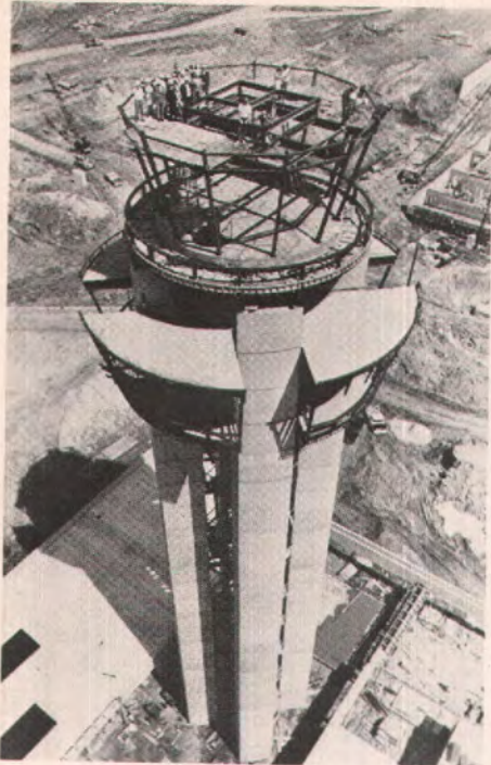
Fig. 1(a). Airport control tower. Structural steel platforms were set at 15-ft (4.57 m) intervals to connect the four service cores.
