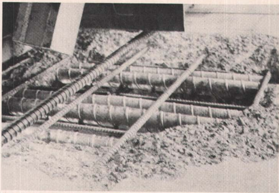
Fig. 5. Longitudinal ducts spaced too closely.
