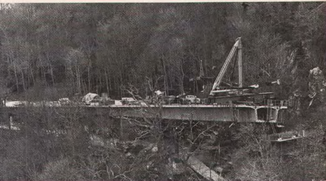
Fig. 1. Linn Cove Viaduct constructed with precast segments erected by progressive placing. This photo shows progress through February 1982.
