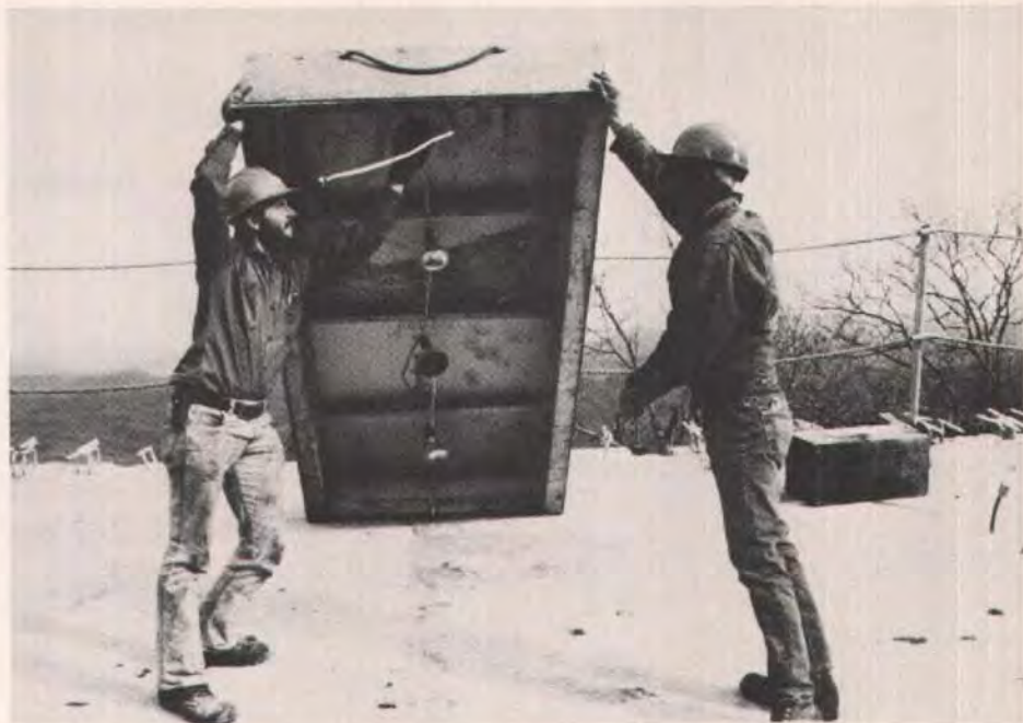
Fig. 7. Heating box, built with plywood and insulated with styrofoam, for heating the top of the joint.
