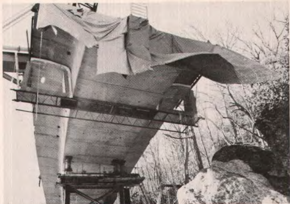
Fig. 6. The foam on the edges of the heating frame provided a good seal as the frame was moved from joint to joint around the curve.
