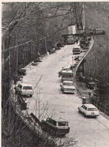
Fig. 2. All substructure and superstructure erection is being done from the top. Here, a precast pier segment is being lifted by the stiffleg crane.
