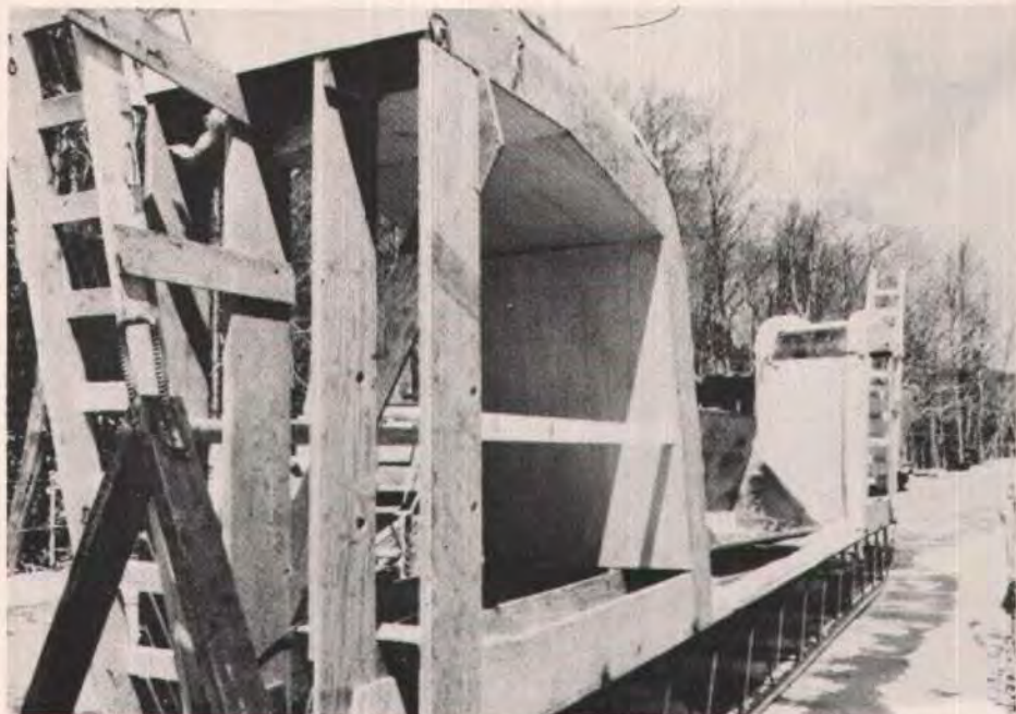
Fig. 5. The insulating frame was built to the general configuration of the outside of the box girder. The out-to-out width is 4 ft (1.2 m).
