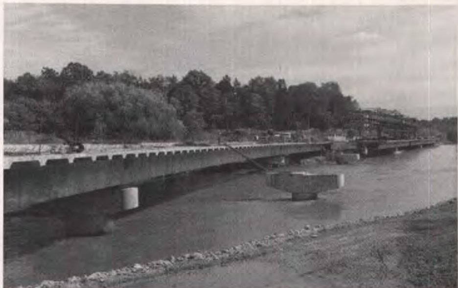
Fig. 7. Completed northbound bridge with southbound bridge under construction. Note mislocated Pier 4 with Pier 5 in the foreground.
