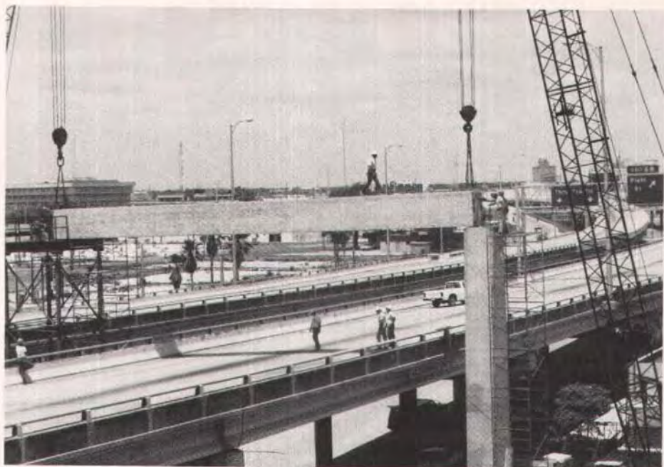
Fig. 7. Traffic was detoured on the Crosstown Expressway while one of the two 70-ft (21.3 m) segments is being erected. Note the temporary bent at the left.
