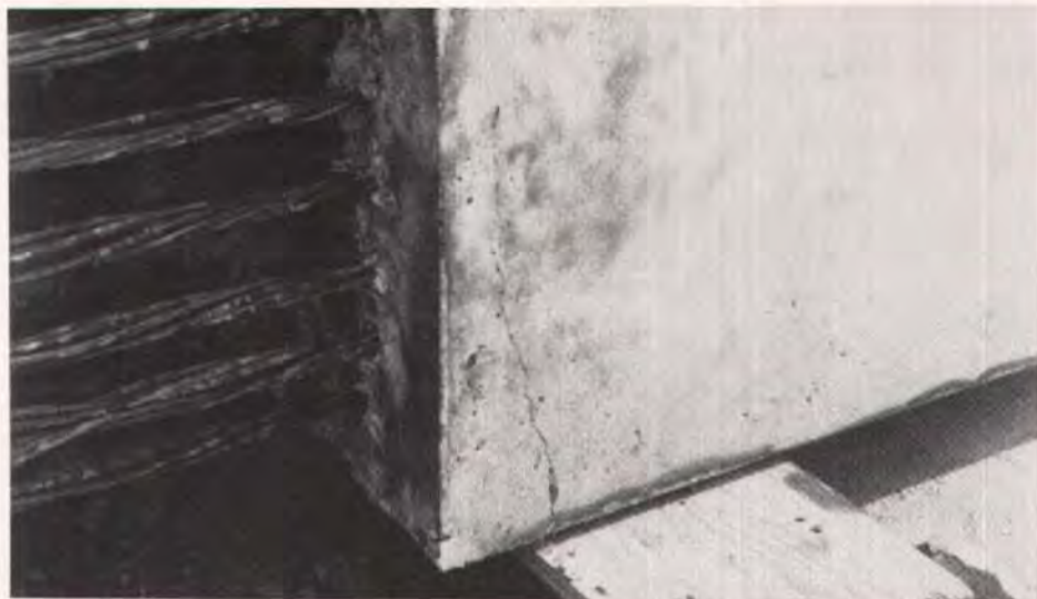
Fig. 10. Bearing failure cracks formed in some of the girders cast early in the project. The cause was quickly identified and a solution to the problem was found.
