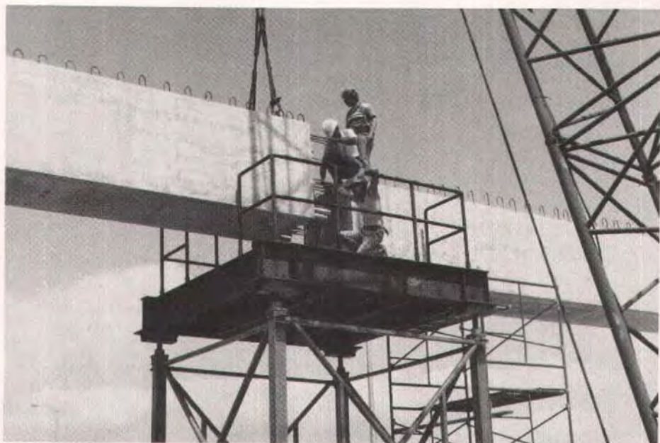
Fig. 8. Closeup view at the temporary support side of the other 70-ft (21.3 m) segment being set into place.
