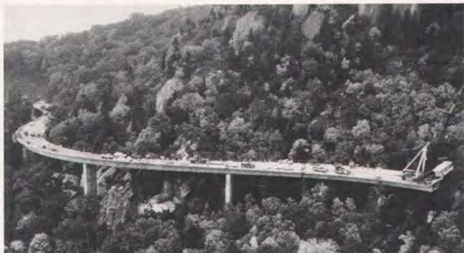
Fig. 2. Construction overview of Linn Cove Viaduct. This bridge is the first segmental structure in the United States to incorporate progressive placing erection.
