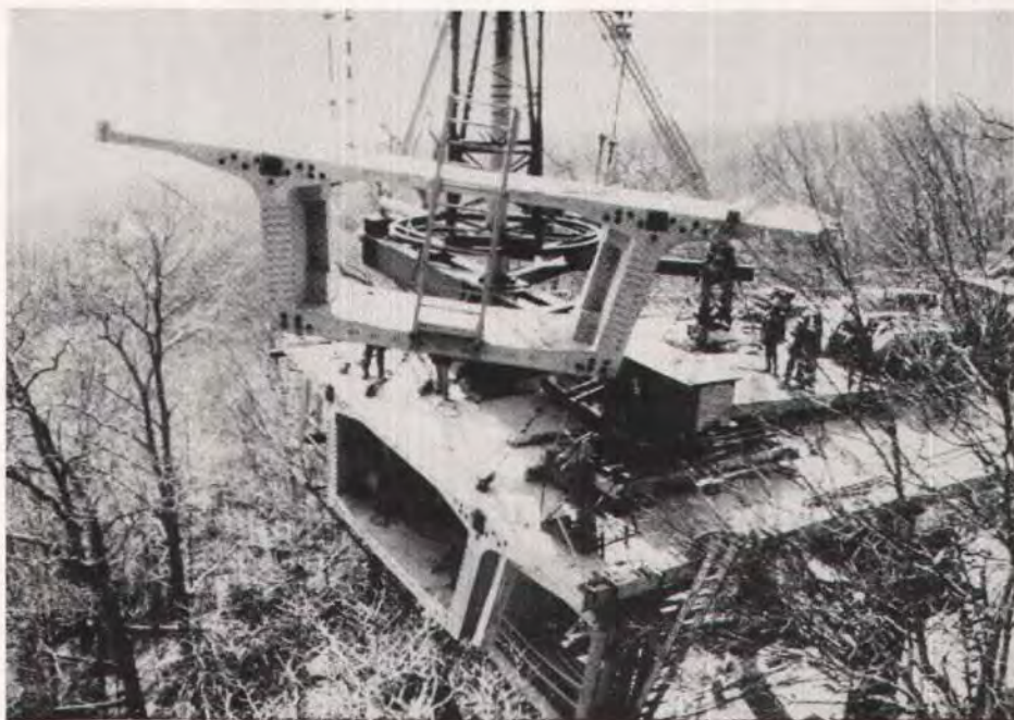
Fig. 12. The segment was lifted from the truck on the right and swung out over the cantilever end.
