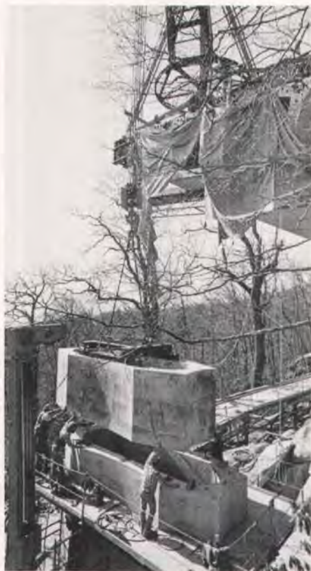
Fig. 9. Precast box pier segments were lowered over the end of the completed cantilever with the stiffleg. The workmen are ready to block the segment and apply the epoxy.
