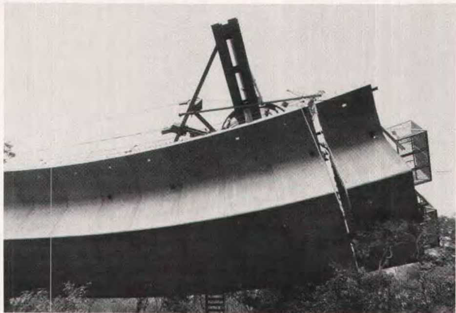
Fig. 14. Here the segment is in place ready to receive the epoxy bonding agent. The excellent fit of the previous joints and the curvature can be seen. Most joints were less than 1 mm (0.004 in.) in thickness.
