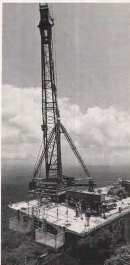
Fig. 8. The contractor chose to erect the segments with this stiffer crane attached to the end of the cantilever. This single piece of equipment controlled the construction rate of the bridge. All material and equipment was handled with this crane.
