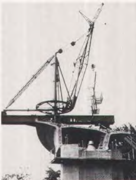
Fig. 11. The first step in the erection sequence was to remove the post-tensioning stressing cage from the end of the cantilever. The permanent tendon live end anchors can be seen at the top of the webs.
