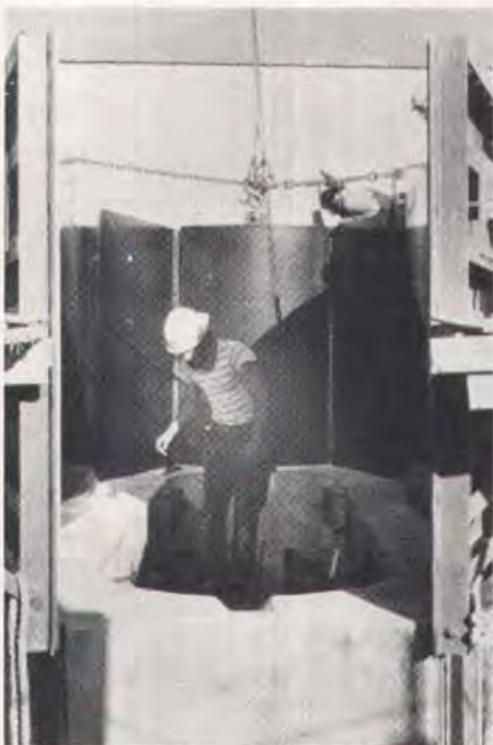
Fig. 6. The box piers were cast with a vertical match-cast system. Here the cast-against segment is being prepared for casting its neighbor on top.
