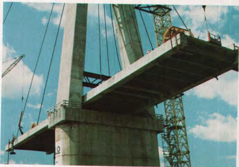
Fig. 4. The southern portion of the bridge was built using cast-in-place segmental cantilever construction and traveling formwork.
