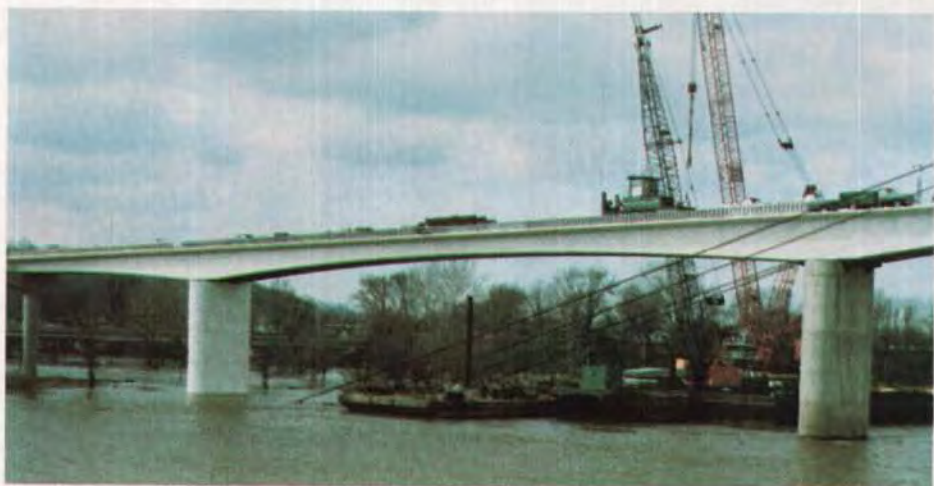
Fig. 10. The 300 ft (91.4 m) segmentally cast end span. Note temporary cables used to stabilize tower girder during erection.
