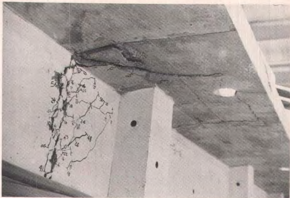
Fig. 12. Joint 4-5 of the Unbonded Tendon Girder after testing.
