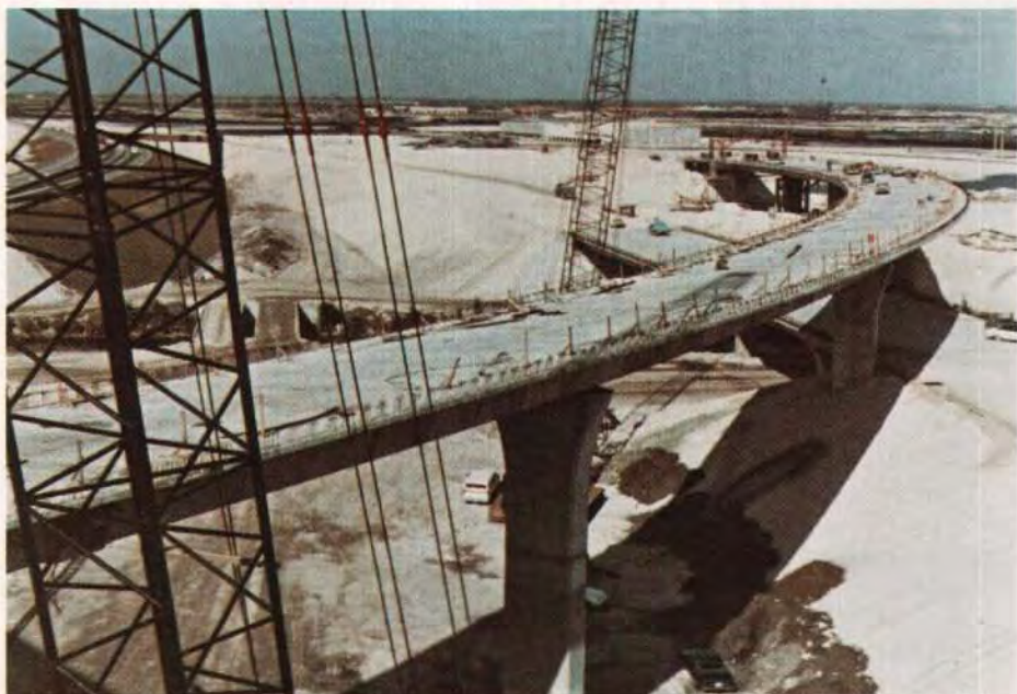
Fig. 18. Segmental cantilever bridges under construction at I75/I595 Phase 2 project. (Contractor: Harbert/Westbrook Joint Venture. Designer: Beiswenger, Hoch and Associates)
