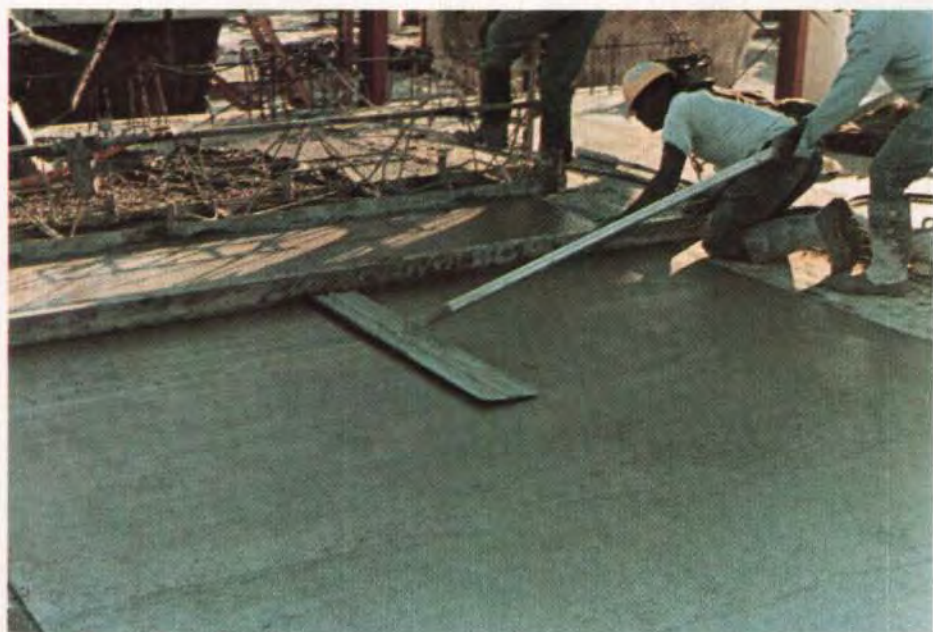
Fig. 17. Use of a vibratory screed, followed by straightedge and light application of bull floats for a good finish.
