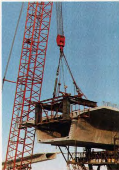
Fig. 12. Balanced cantilever segment erection by crane at US 441/I595 Interchange. (Volker Stevin, Contractor)
