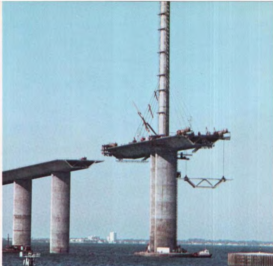
Fig. 14. Main span segment erection at Sunshine Skyway using beam and winch equipment.
