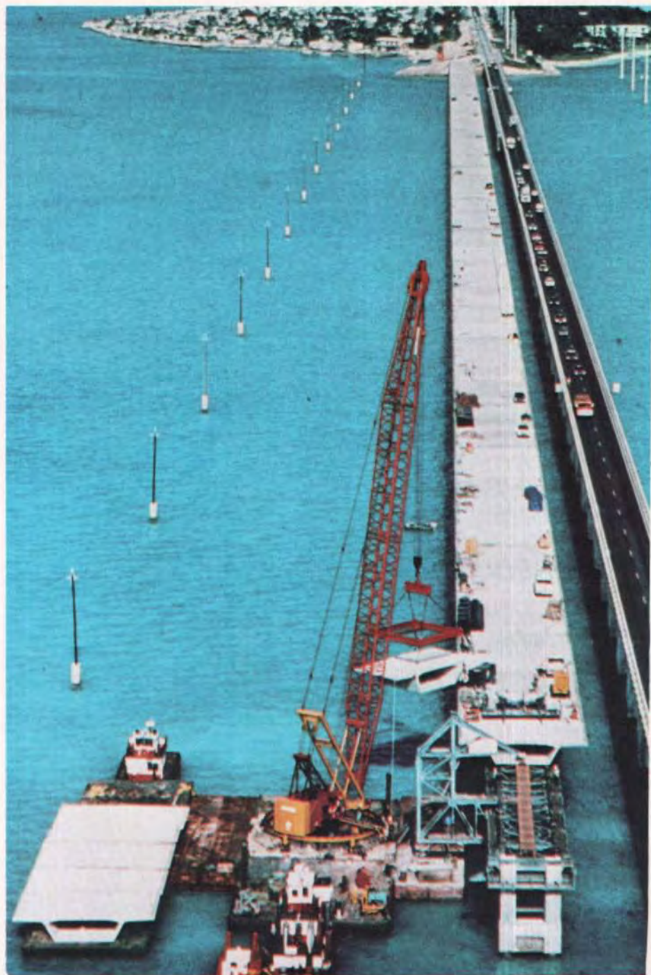
Fig. 1. Long Key Bridge — A precast segmental, post-tensioned, span-by-span structure. (Courtesy of Figg and Muller Engineers Inc., Designer)
