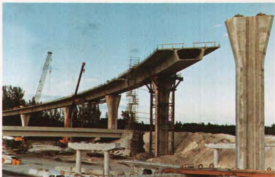
Fig. 15. Balanced cantilevers under construction at US 441/I595 Interchange. (Designer: Greiner Engineering Sciences Inc.)
