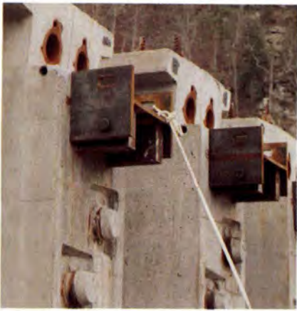
Fig. 18. Cazaly hangers in pier segment end blocks are ready to support drop-in segments.
