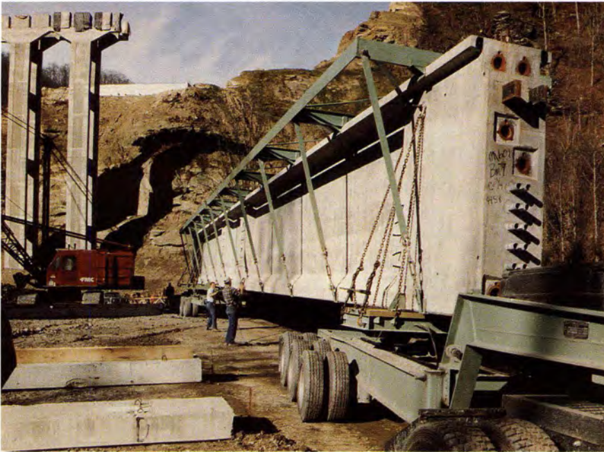
Fig. 14. Special trailer and stabilizing frame used to haul 108 ft (33 m) bridge beams.
