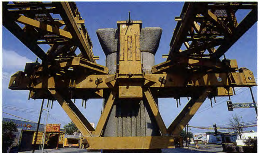
Fig. 20. Erection trusses are supported on steel brackets suspended from and clamped to the piers.
