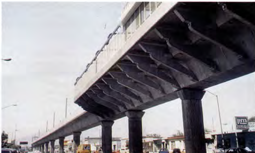
Fig. 24. In the platform areas, precast concrete cross beams are attached to the box girder segments.
