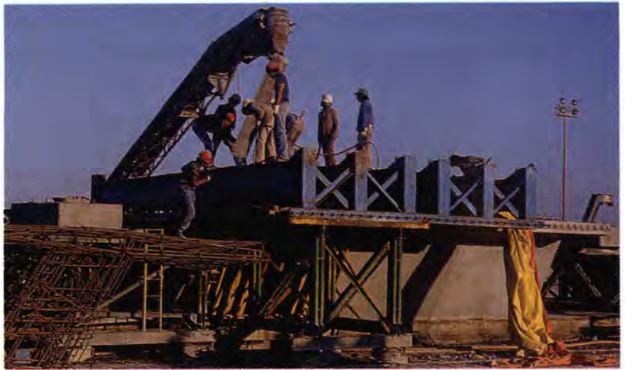
Fig. 13. A segment casting using a conveyor belt to move concrete from truck mixer to mold.
