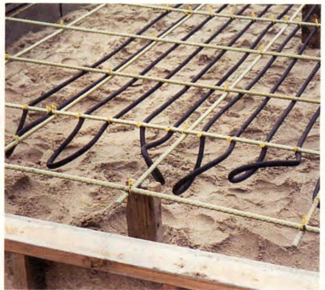
Fig. 11. Deck heating system on approaches.
