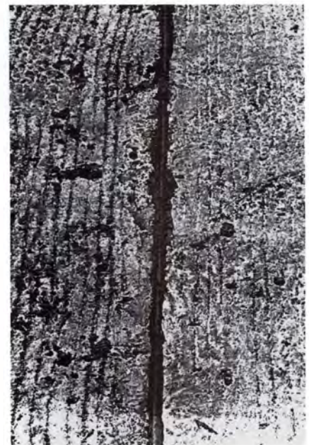
Fig. 16. Gapped joint in segment.
