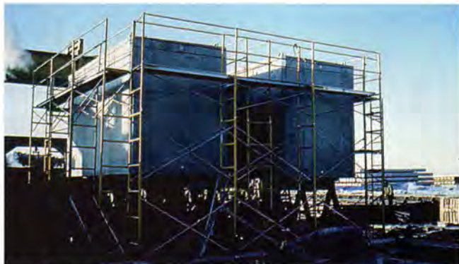
Fig. 8. Box pier segments had a one-day casting cycle. A total of ten segments were produced in a 5-day work week, using two forms.
