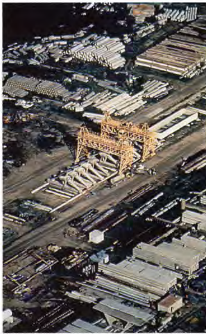
Fig. 7. Overall view of the precasting yard showing various precast components being prepared for shipment to the bridge site.
