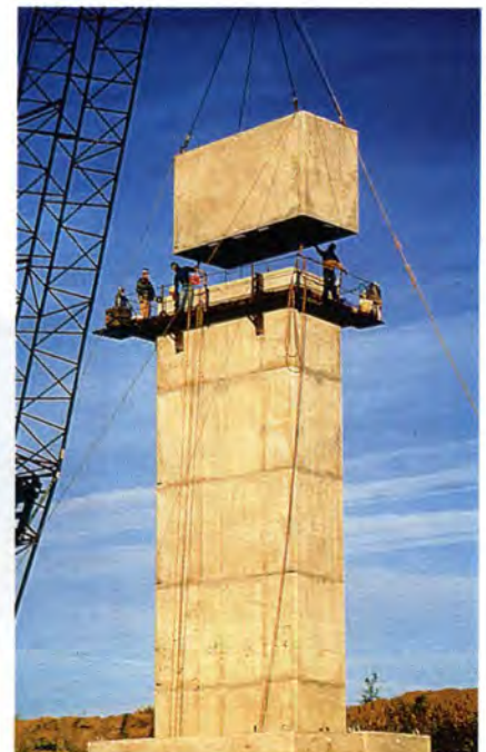
Fig. 11. One of the 463 match cast box pier segments being placed. After setting the last segment in place, the entire precast unit was vertically post-tensioned.
