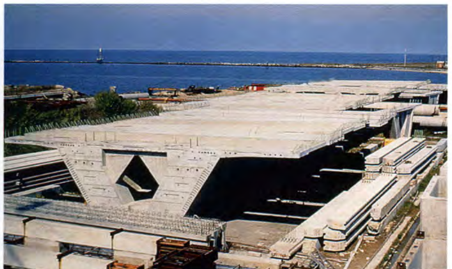
Fig. 12. Special superstructure segments were designed to rest on the precast post-tensioned piers.
