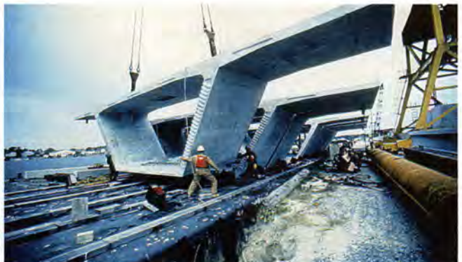
Fig. 9. Trapezoidal box girder segments were match cast to ensure tight tolerances during erection. In all, 984 such girder segments were fabricated.
