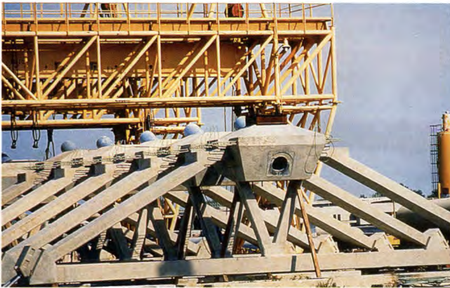
Fig. 10. Precast delta frames were designed to tie the main span box girder segments together and provide anchorages for the cable stays.
