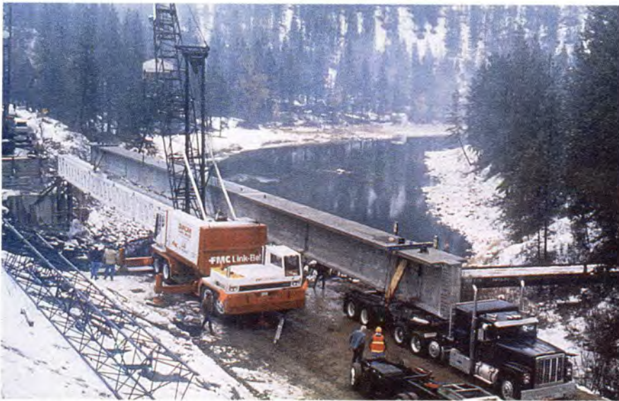
Fig. 19. At bridge site, end of girder placed on launcher trolley and pushed across by truck unit.
