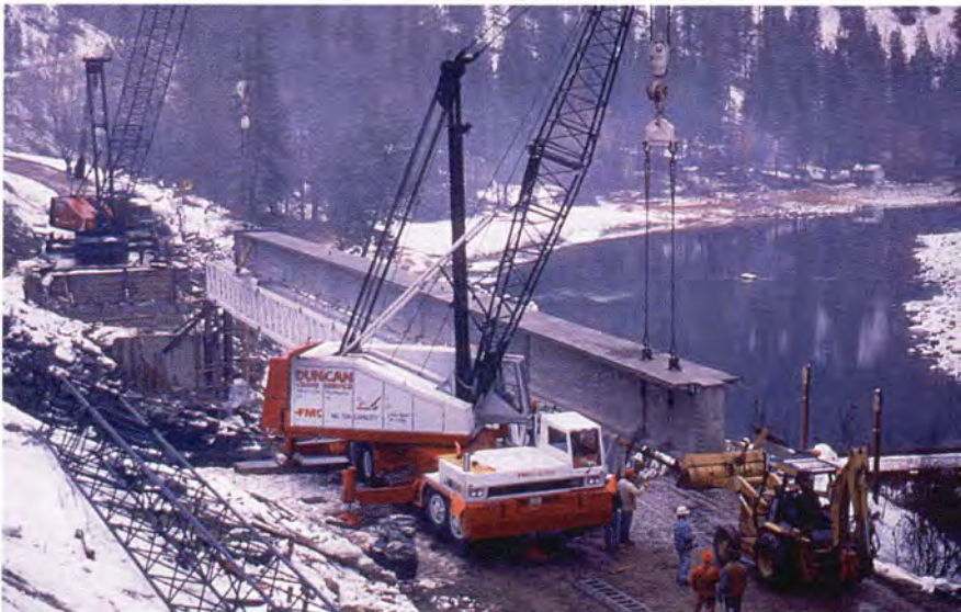
Fig. 20. Girder, weighing 120 tons (110 t), being lifted by a 200 ton (180 t) crane at one end and a 140 ton (127 t) crane at the other end.
