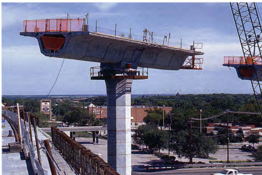
Fig. 17. U.S. 183 Viaduct, Austin, Texas, view of balanced cantilever construction (Designer: Texas Department of Transportation).
