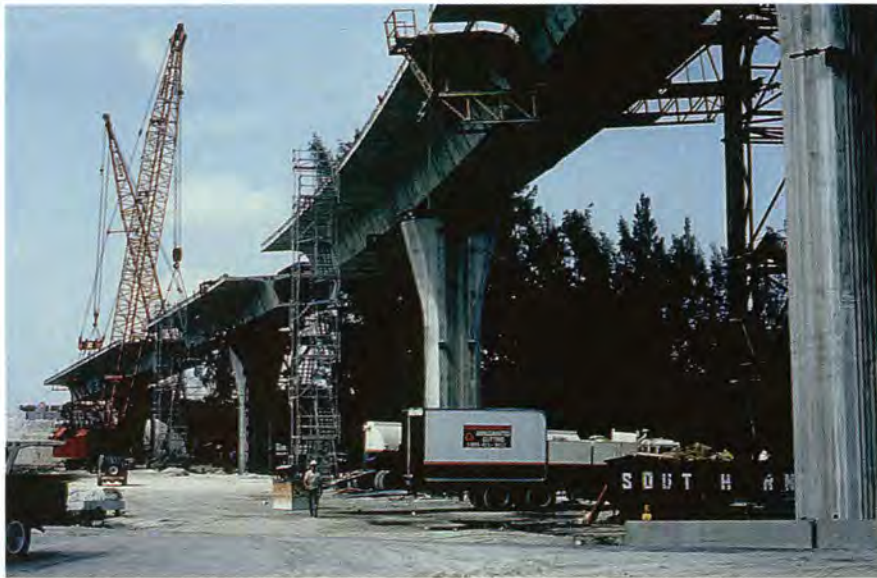
Fig. 5. Balanced cantilevers under construction at U.S. 441/I-595 Interchange (Designer: Greiner Engineering Sciences, Inc.).
