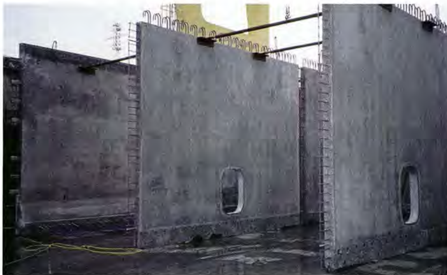
Fig. 12. Erected interior walls showing doorway openings and projected reinforcing bar around edges.
