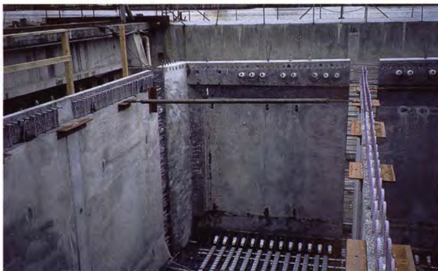
Fig. 13. Erected corner cell. Note reinforcing bar couplers at top of exterior wall at left.
