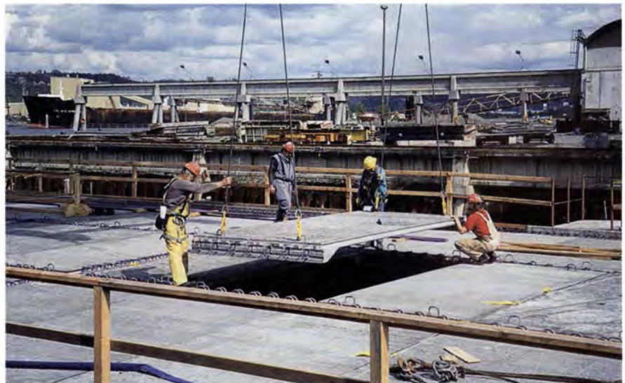
Fig. 20. Erecting haunched deck panels used as stay-in-place forms for the pontoon top slab.
