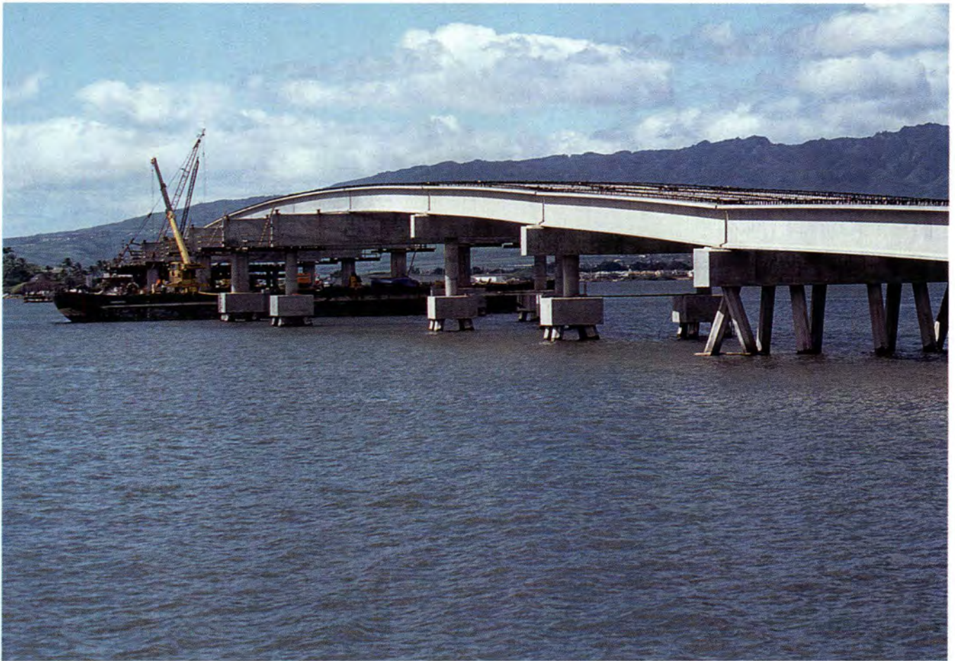
Fig. 3. Fixed approach spans comprising continuous prestressed bulb-tee girders and deck panels supported on pile bents and caps, and prestressed piles.
