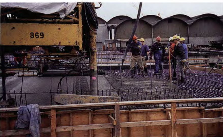
Fig. 24. Pouring a silica fume concrete overlay on the channel beams and the 9 in. (229 mm) roadway slab.
