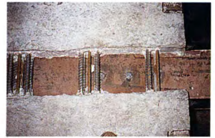
Fig. 12. Precast panels in place over girder lines showing large space available for placement of connector with reinforcement (see Fig. 13 below).
