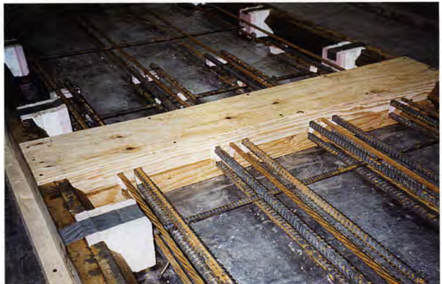
Fig. 9. Forming of gap at girder line.
