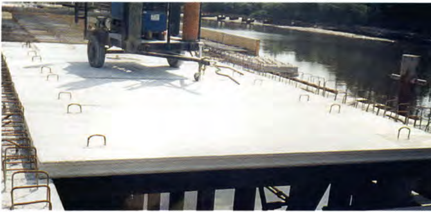
Fig. 9. Precast slabs are installed over precast beams. The prestressing strand is left exposed 12 in. (305 mm) at both ends of the slab, providing the anchorage with positive reinforcement.
