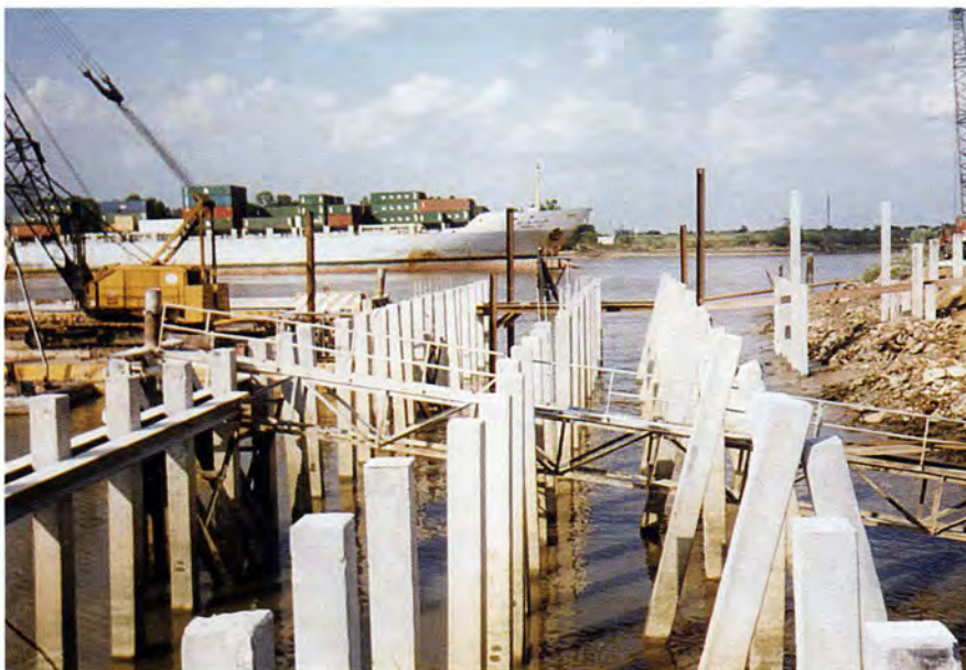
Fig. 4. Precast piles are driven by barge crane. A temporary steel beam template is installed as a guide for driving the piles. A walkway bridge to barge and breasting dolphin was also temporarily installed.
