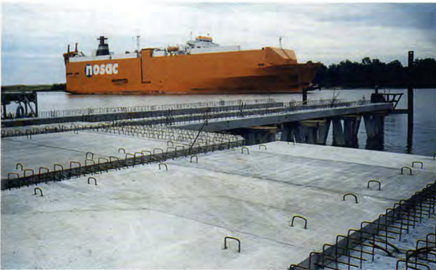
Fig. 10. Precast slab provides an instant working platform, thereby eliminating the need for forming and placement of reinforcing steel over water.
