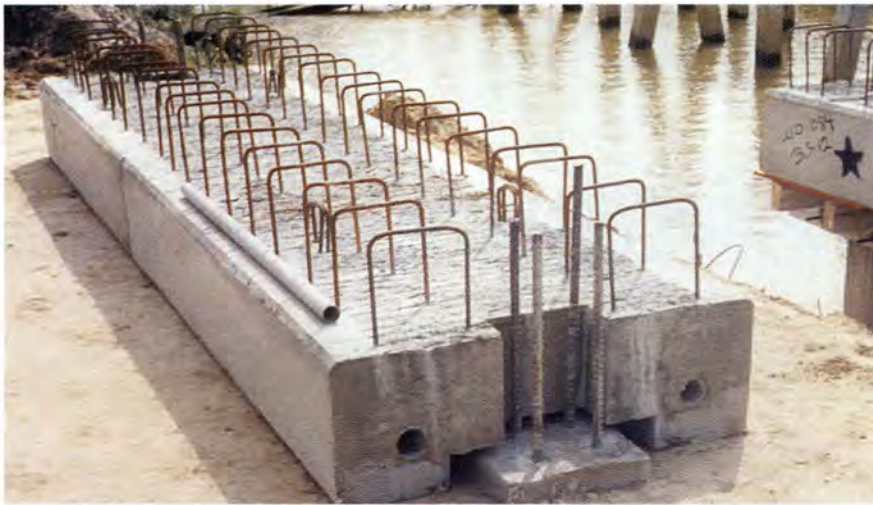
Fig. 7. Positive reinforcement is spliced at the grout to be embedded in the precast beam. Steel dowels tie the connection together.
