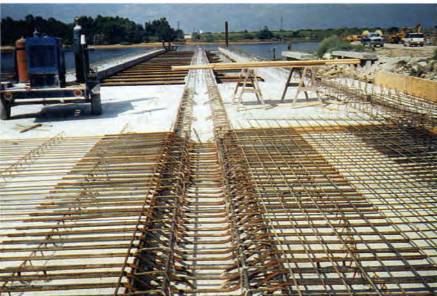
Fig. 11. Negative reinforcement is placed over the precast beam and precast slab, with 8 in. (203 mm) of cast-in-place concrete over the reinforcing bars.
