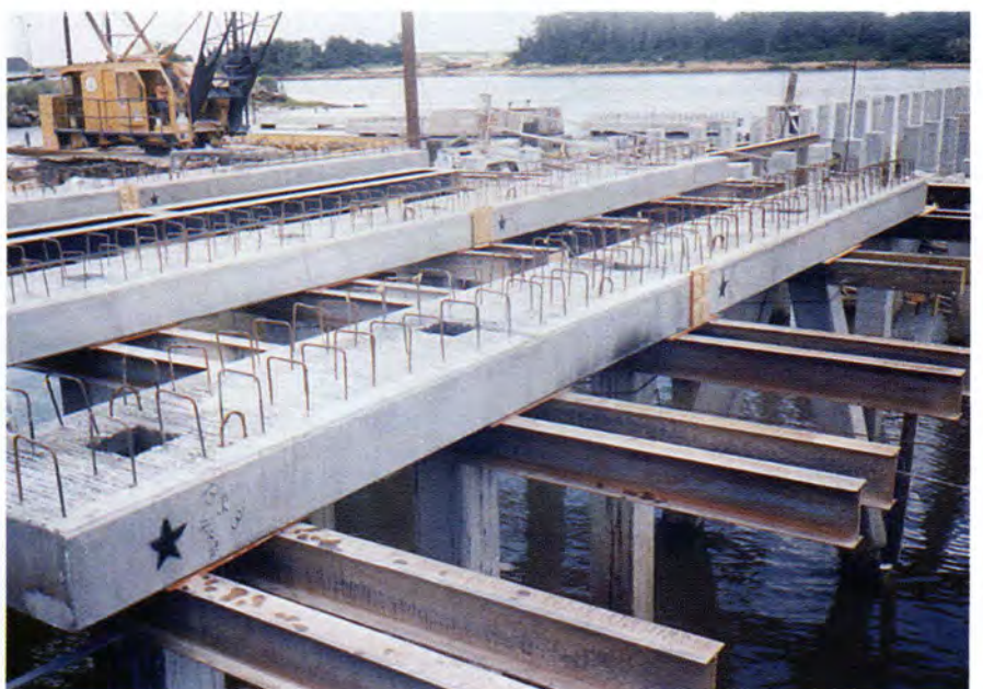
Fig. 6. Simple span beams are field-connected into multiple span continuous beams. Beams are spliced at approximately every three spans, over the pile cap.
