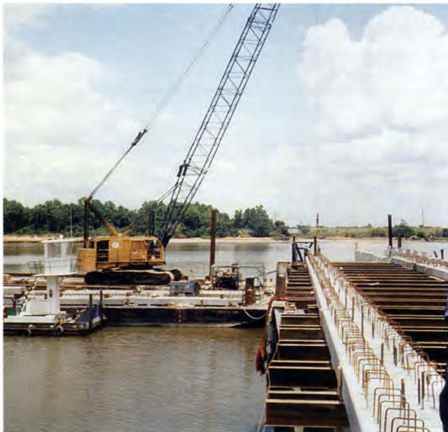
Fig. 8. The barge crane and tug boat has to be off the navigation channel when a ship arrives. The precast erector seizes the opportunity to install precast beams in the time allotted.
