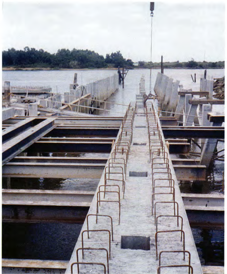
Fig. 5. Precast beams are installed into the tops of piles. Note that steel beam templates provide the true plumb and square to the specified location.
