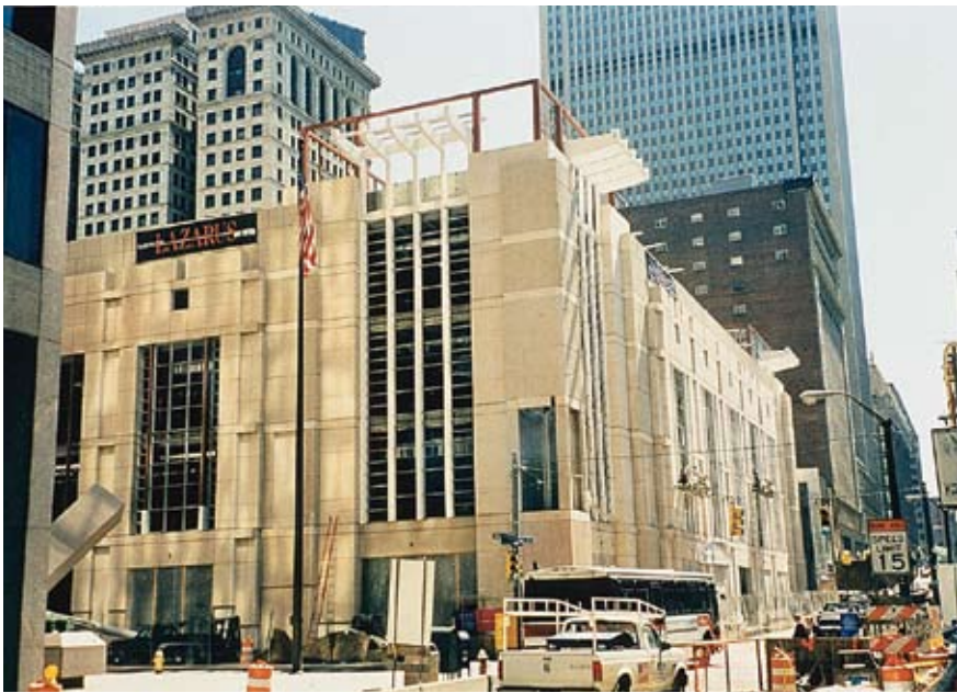
Fig. 11. Erection of the panels required both a day and night crew, with major challenges arising from having to work in the busy downtown area.
