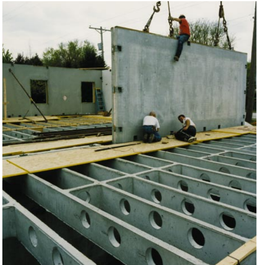
Precast concrete flooring consists of longitudinal panels spaced 2 feet apart, which provided spans up to 40 feet in the basement.
