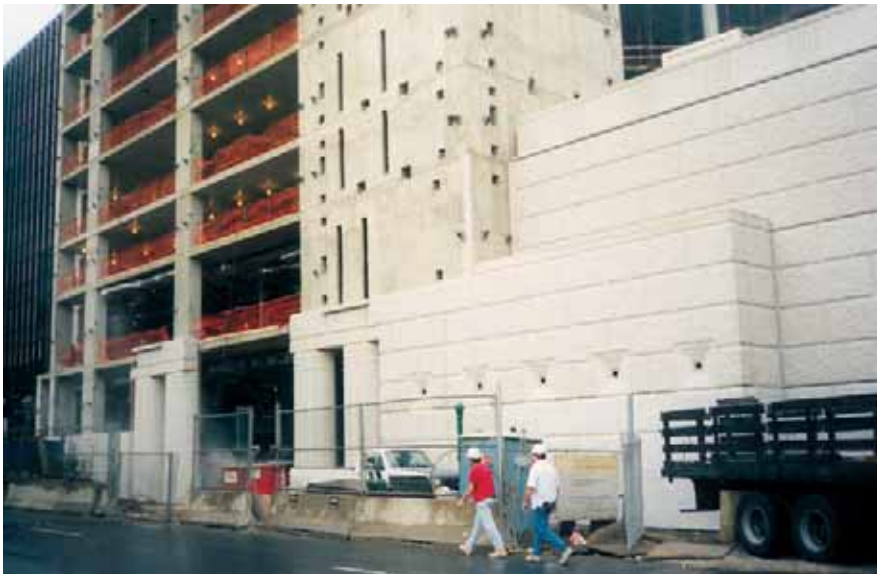
Fig. 18. Shear walls with blockouts were included for connection to precast panels. Photo courtesy: Jeffrey Totaro.
