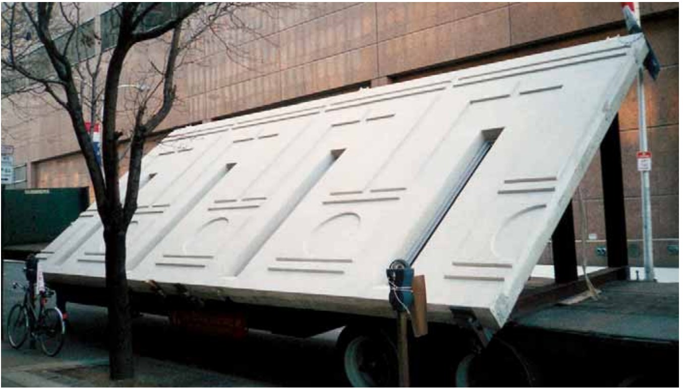
Fig. 16. With a downtown urban site and a building filling the available footprint, precast panels remained on the trucks until they could be erected that night. Photo courtesy: Jeffrey Totaro.
