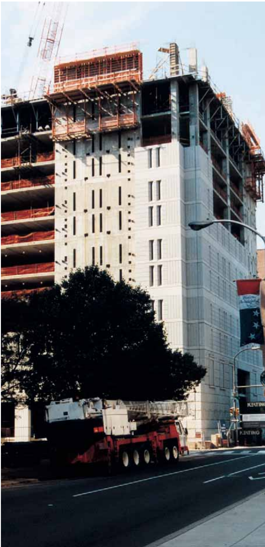
Fig. 20. Erection was performed with the crane located within the perimeter of the building due to the constrained downtown site. Photo courtesy: Robert Meier.
