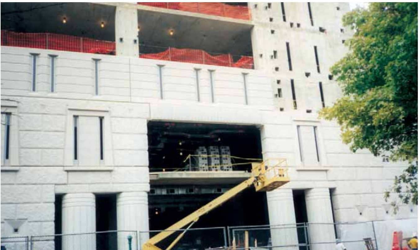
Fig. 19. One bay of precast panels was left open to allow for construction access after the rest was finished. Photo courtesy: Jeffrey Totaro.
