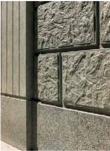
Fig. 7. Form liners and polishing achieved these dramatically different panel textures. Photo courtesy: Robert Meier.
