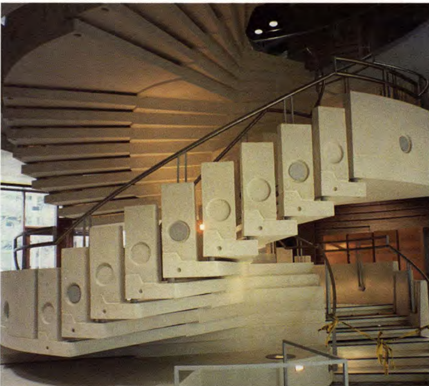
Fig. 19. Adding complexity to the calculations was the decorative precast guardrail on the end of each tread, which added more weight to each cantilevered segment.
