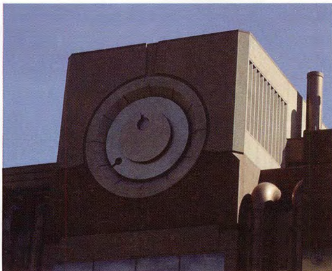
Fig. 12. The precast "atomic clock" was created with five support panels for hauling and erection.
